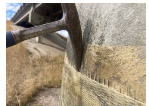
Bridge #02096, random delamination of FRP repair
