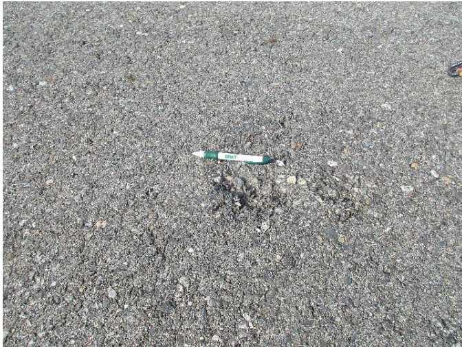
T-1 , Surface detail with raveling
