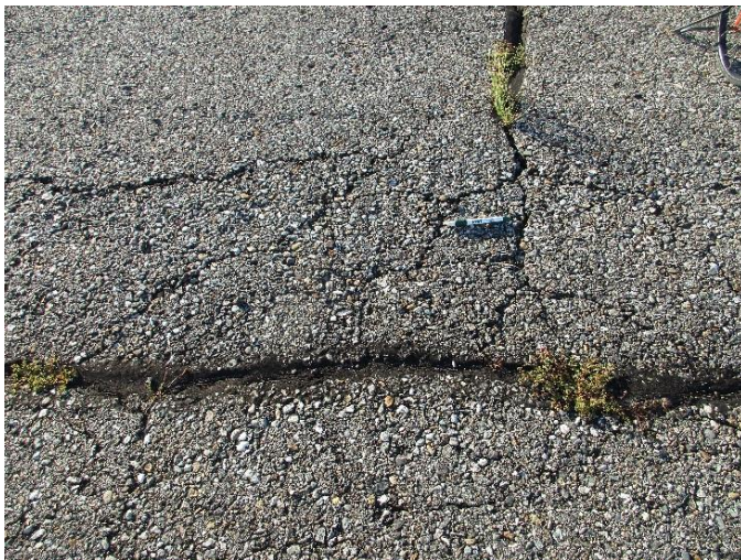
A-2, Surface detail with alligator cracking
