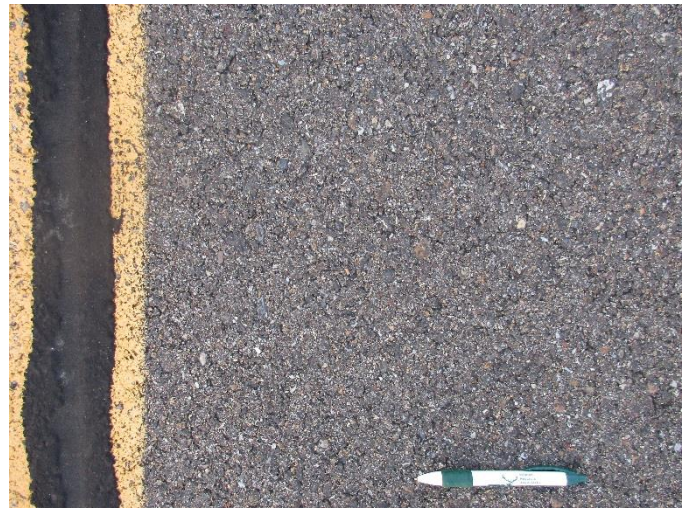
T-5, Surface detail with sealed crack
