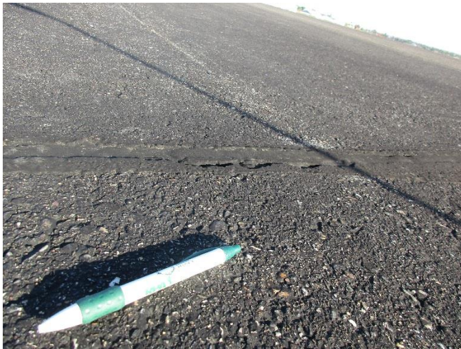
T-1, Surface detail with raveling
