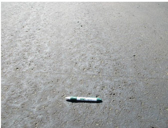
T-5, Surface detail with bleeding
