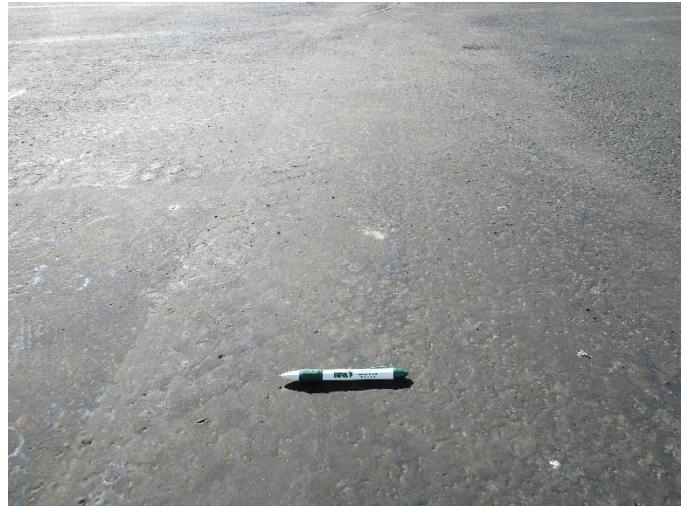
A-1, Surface detail with bleeding
