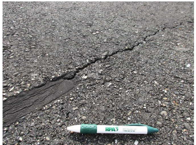
T-1 , Surface detail with low cracking
