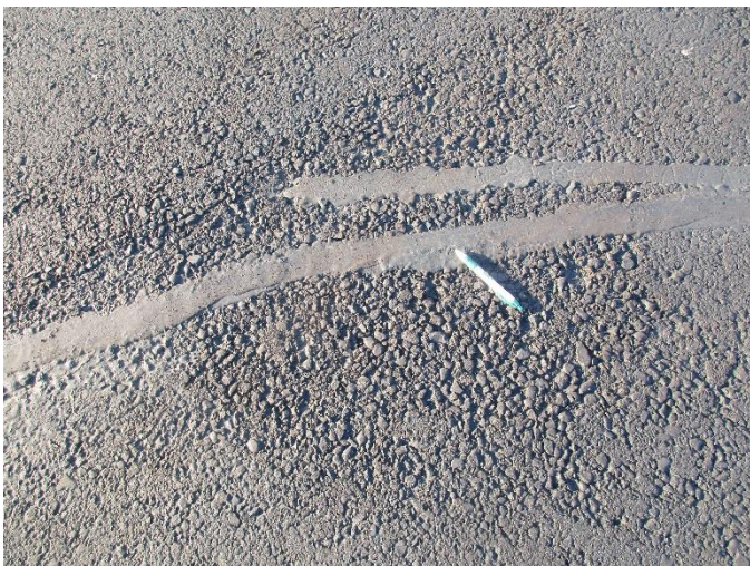
T-1, Surface detail with crack
