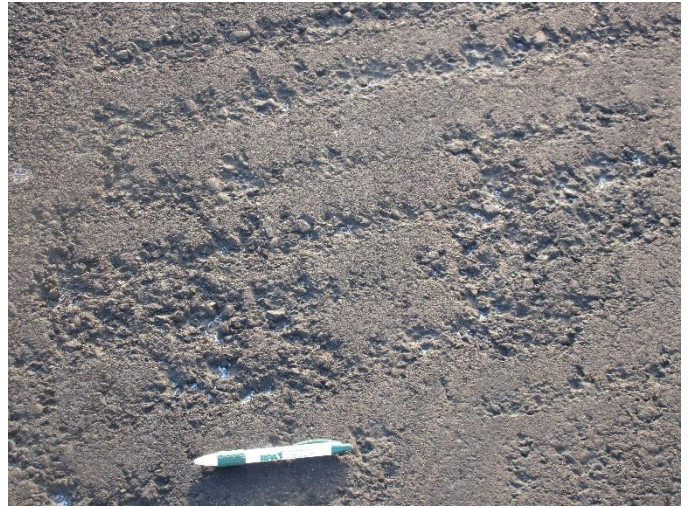
R-1, Surface detail with raveling / gouge
