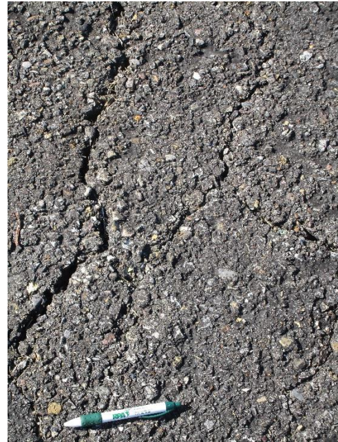
T-4, Surface detail with cracking
