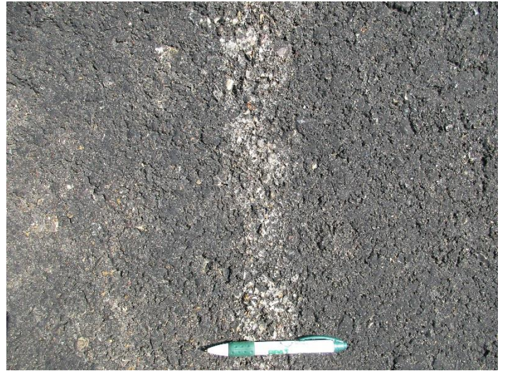
R-2, Surface detail with raveling
