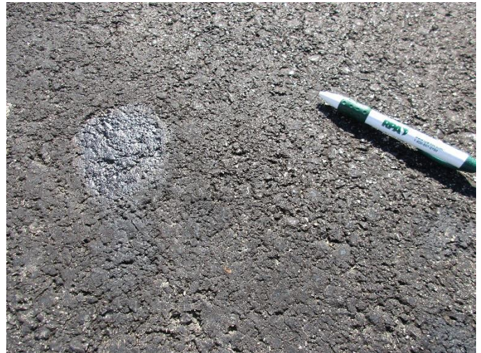
A-5, Surface detail with oil spillage
