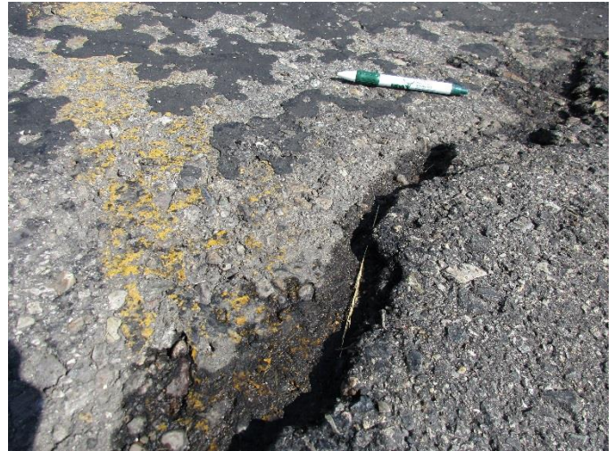
T-2, Surface detail with cracking
