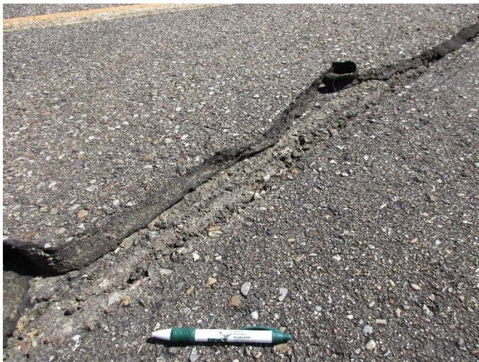
T-1, Surface detail with failed crack sealant
