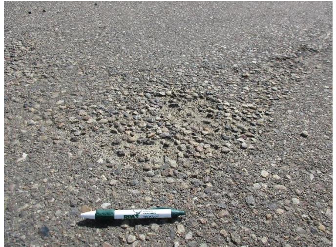
A-1, Surface detail with raveling
