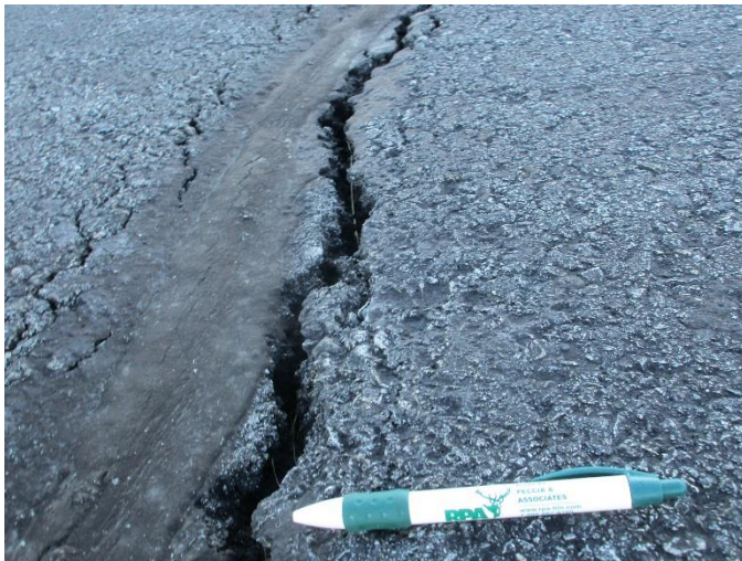
T-1 , Surface detail with cracking
