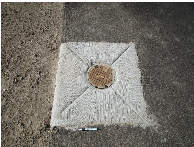
R-15 , Surface detail with concrete patch
