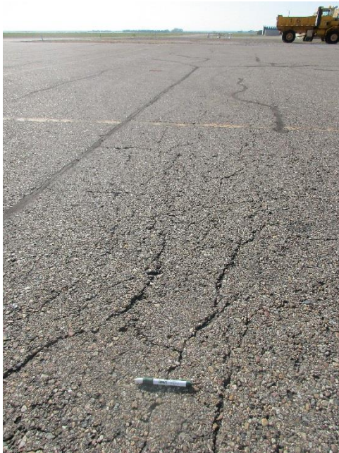
A-5 , Surface detail with alligator cracking
