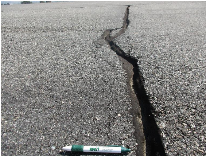
R-4, Surface detail with cracking
