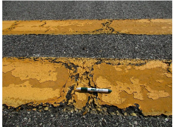
T-8, Surface detail with crack and striping
