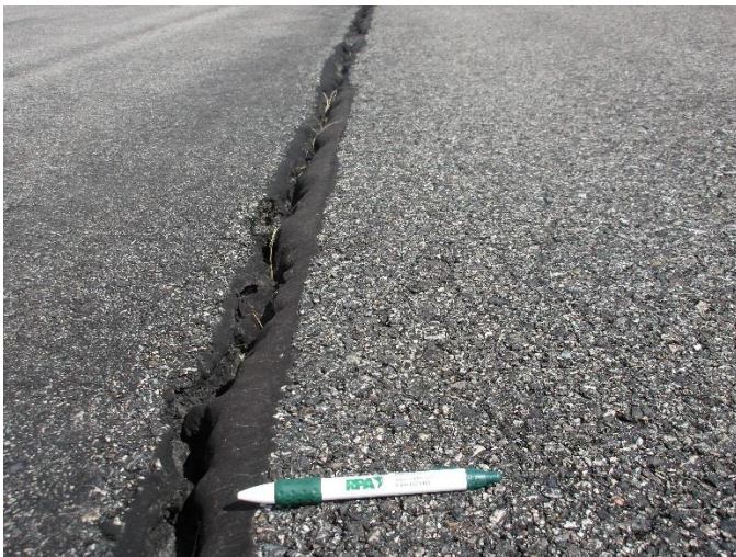
T-9, Surface detail with failed sealant
