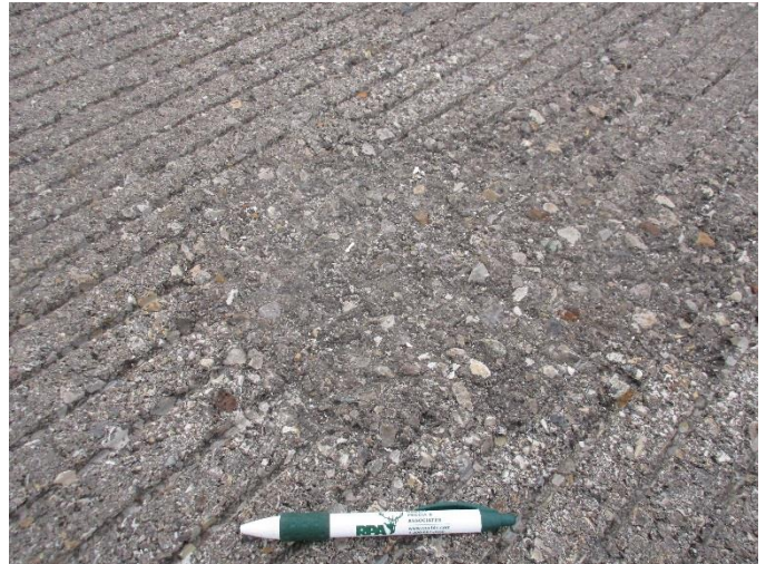
R-34, Surface detail with raveling
