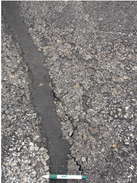
T-8, Surface detail with cracking
