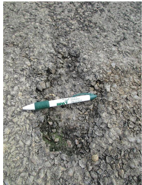
T-1, Surface detail with high raveling
