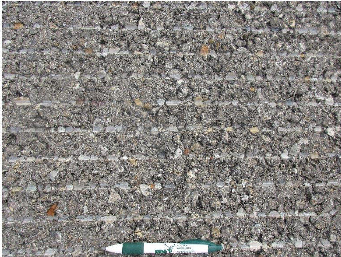
R-32 , Surface detail with grooves
