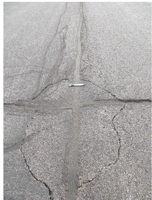
R-23, Surface detail with cracking
