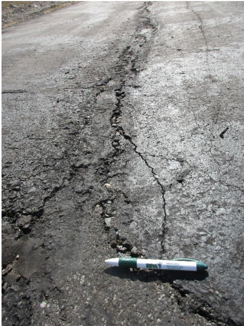
T-2, Surface detail with cracking
