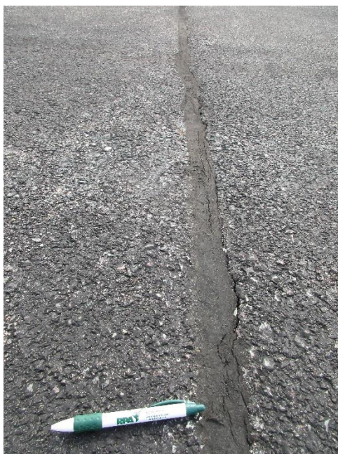
A-3, Surface detail with cracking
