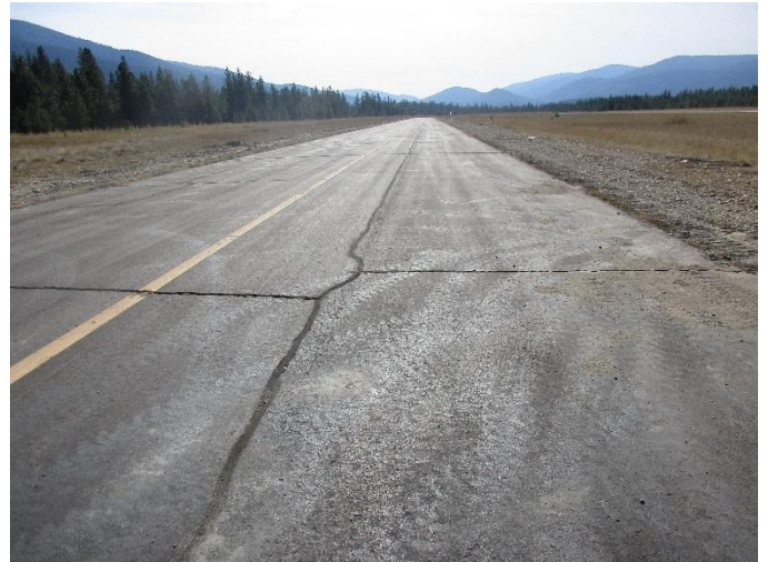
T-2, Overview with cracking
