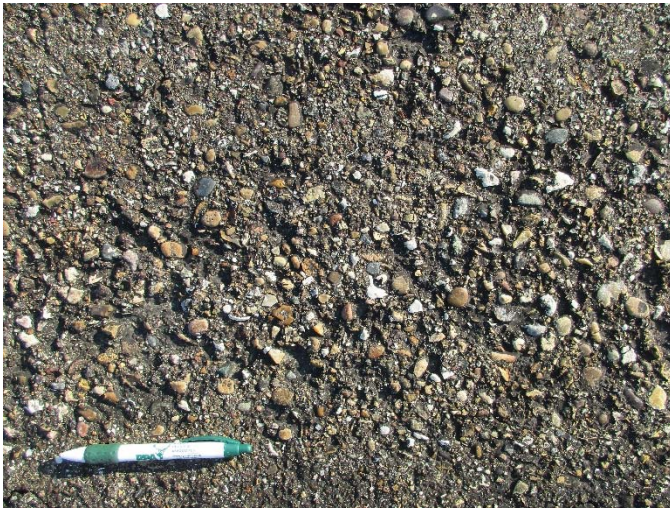
R-11 , Surface detail with raveling
