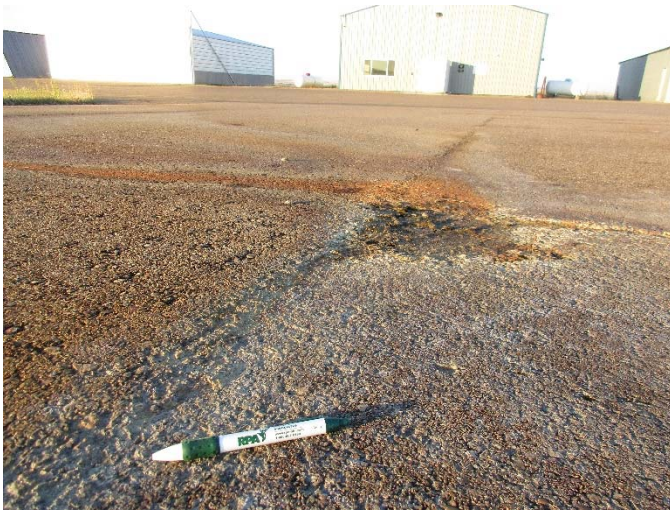
A-11 , Surface detail with depression & staining
