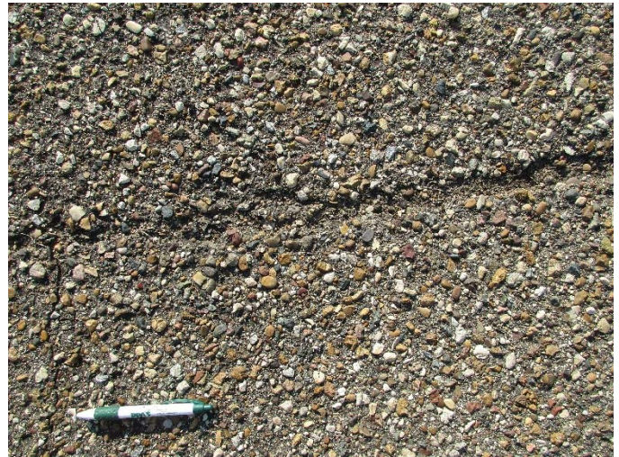
T-11 , Surface detail with a crack and weathering
