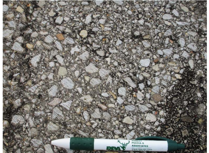
T-1, Surface detail of aggressive paint removal
