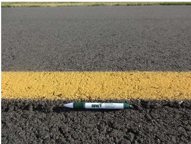
T-4, Surface detail with cracking
