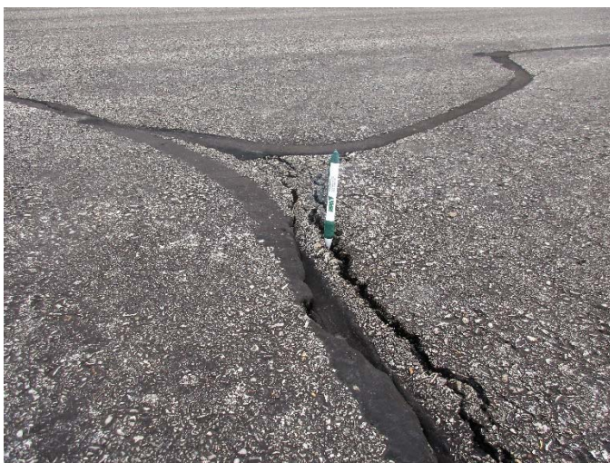
R-1, Surface detail with cracking
