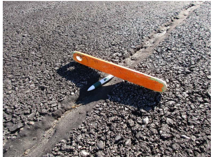
R-3, Surface detail with depression at crack
