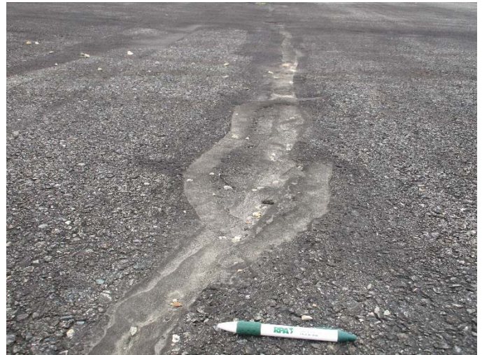
A-2, Surface detail with sealed cracks
