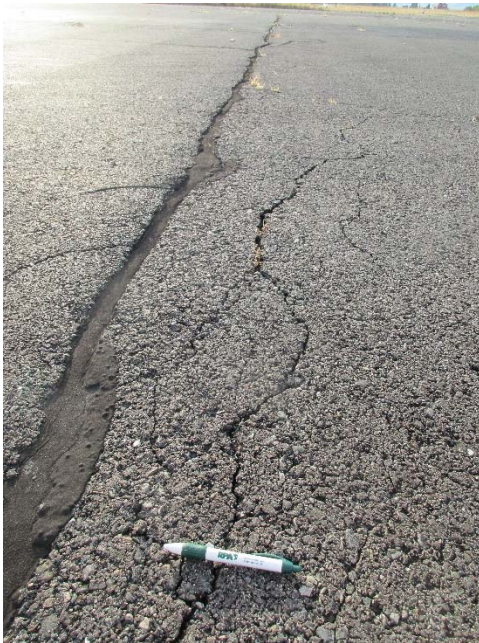
A-2, Surface detail with cracking
