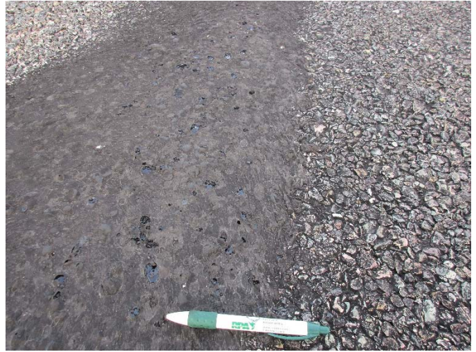
R-1 , Surface detail with bleeding
