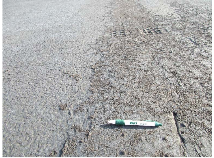
A-1, Surface detail with bleeding
