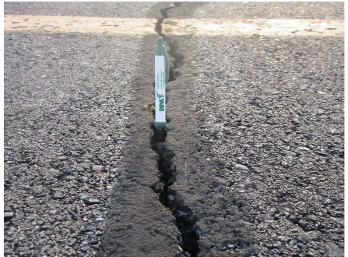
T-3 , Surface detail with cracking
