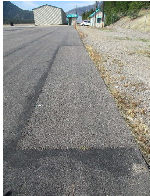
A-11 , Surface detail with patch
