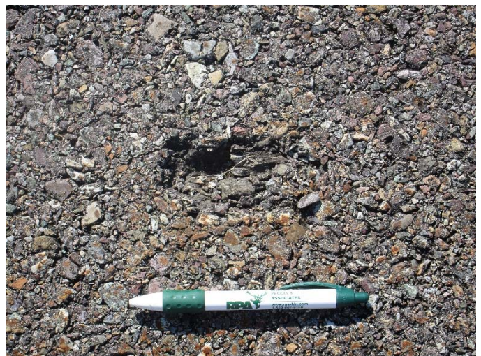
R-11 , Surface detail with raveling (wooden survey hub pushed up through pavement)
