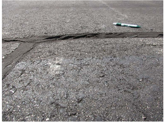
A-1 , surface detail with cracking
