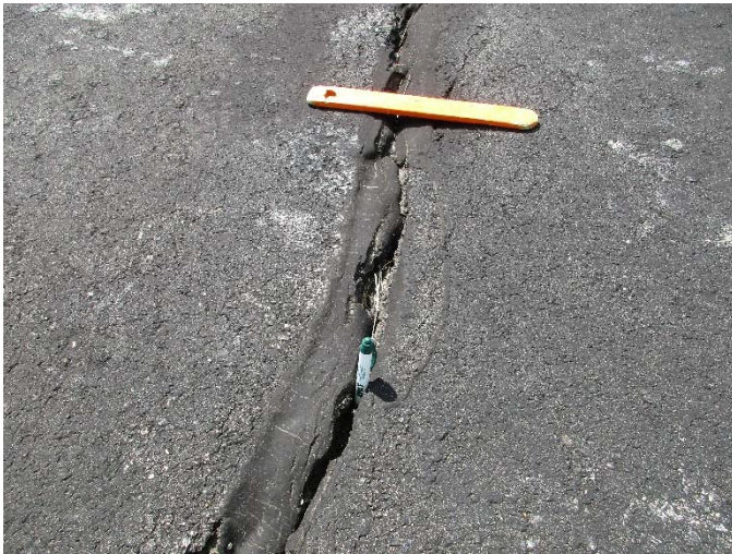
R-1 , surface detail with cracking
