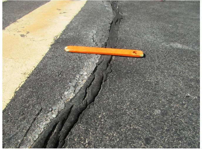
T-1 , surface detail with cracking & raveling
