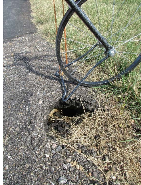
T-3 , Surface detail with raveling & depression
