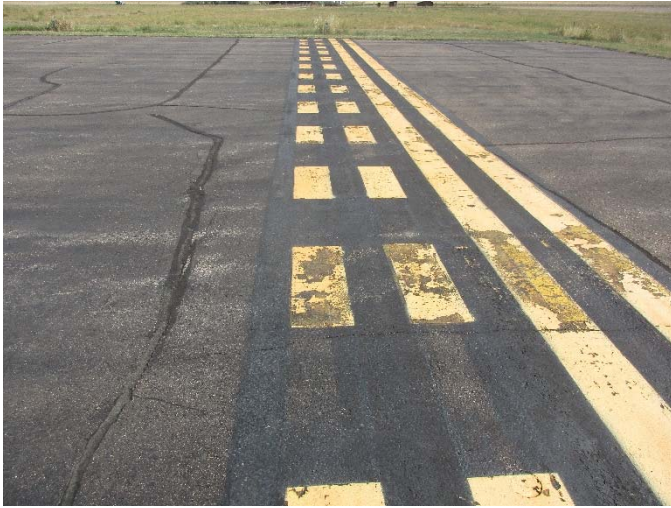
T-3 , Overview with cracks, weathering, & raveling
