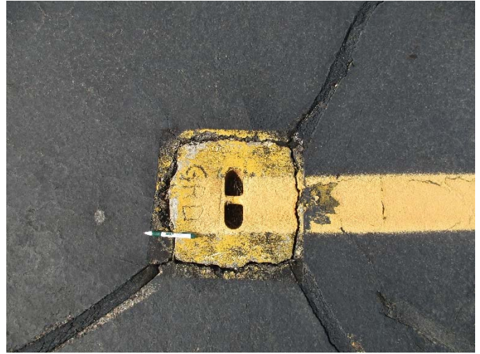
A-1 , Surface detail with cracks & patch
