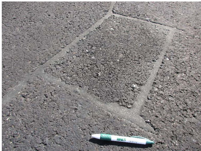
A-11 , Surface detail with patch & sealed cracks
