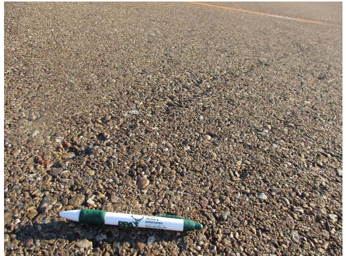
A-5, Surface detail with raveling/gouge
