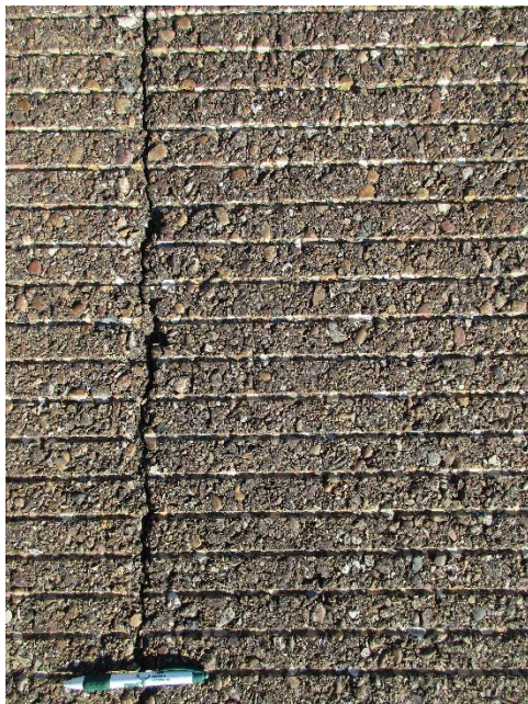
R-11, Surface detail with crack & weathering
