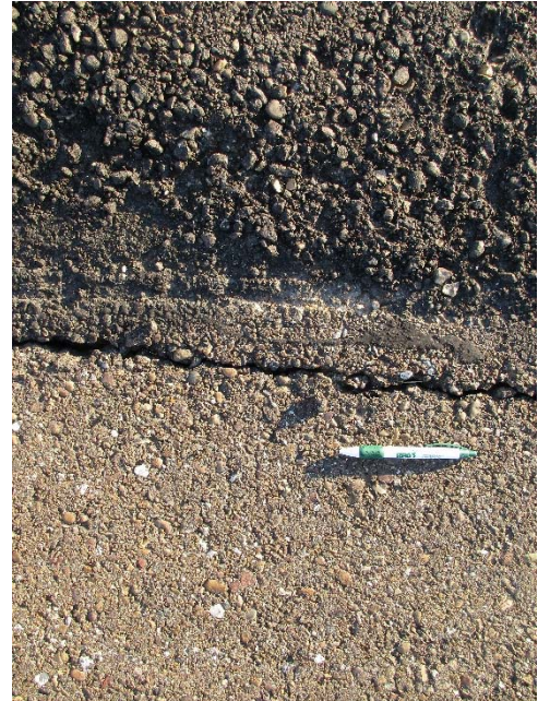
T-4, Surface detail with crack & raveling
