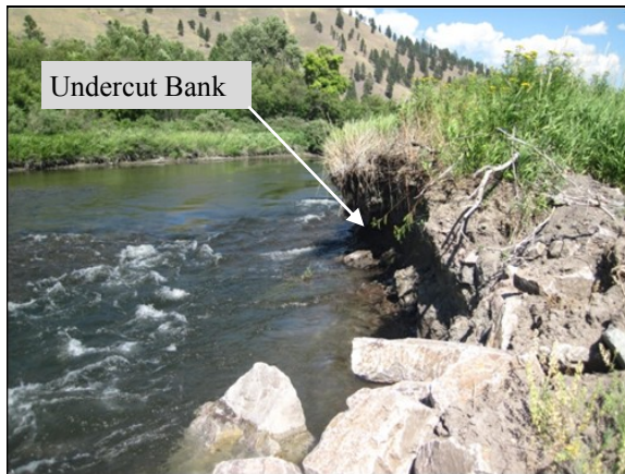
Photo 7 Description: Eroding streambank at upstream extent. Taken in 2013
