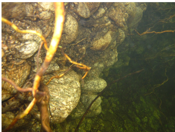
Photo 3 Description: Underwater photo of large hole downstream of project site.
