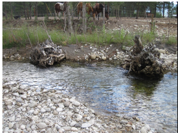
Photo 2 Description: Root wad upstream of bridge showing scour.
