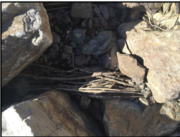
Additional Photo 1 Description: Dead willows in revetment Taken in 2016
