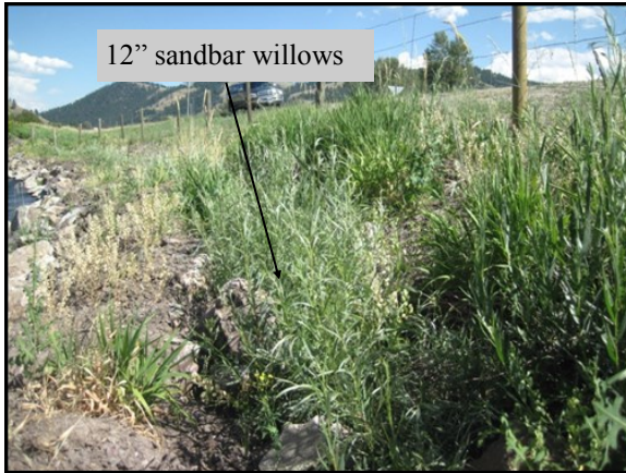
Photo 4 Description: Willow growth at top of revetment. Taken in 2013
