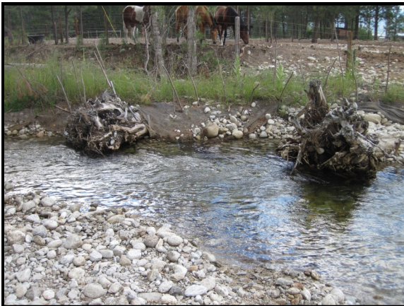
Additional Photo 2—2014 Description: Root wad upstream of bridge showing scour.
