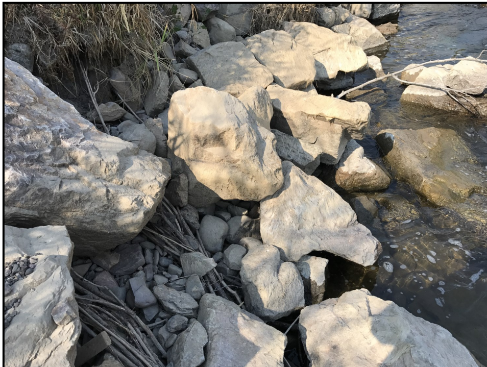
Additional Photo 2 Description: Dead willows in revetment Taken in 2017
