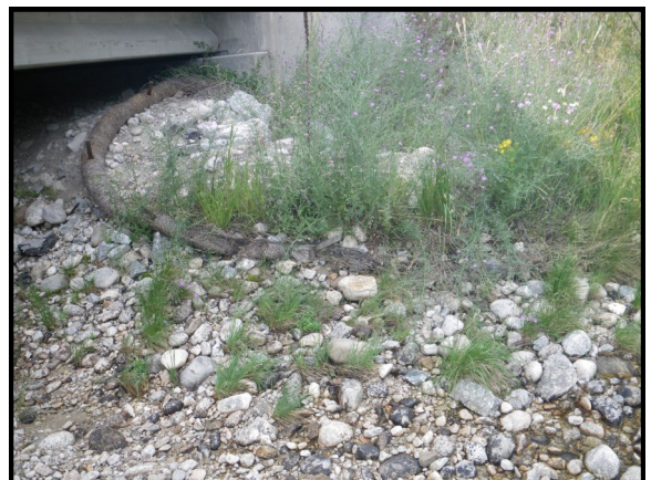
Additional Photo 6: Looking at the left bank downstream of the bridge at a wattle that was installed as a part of utility installation project has become exposed.
