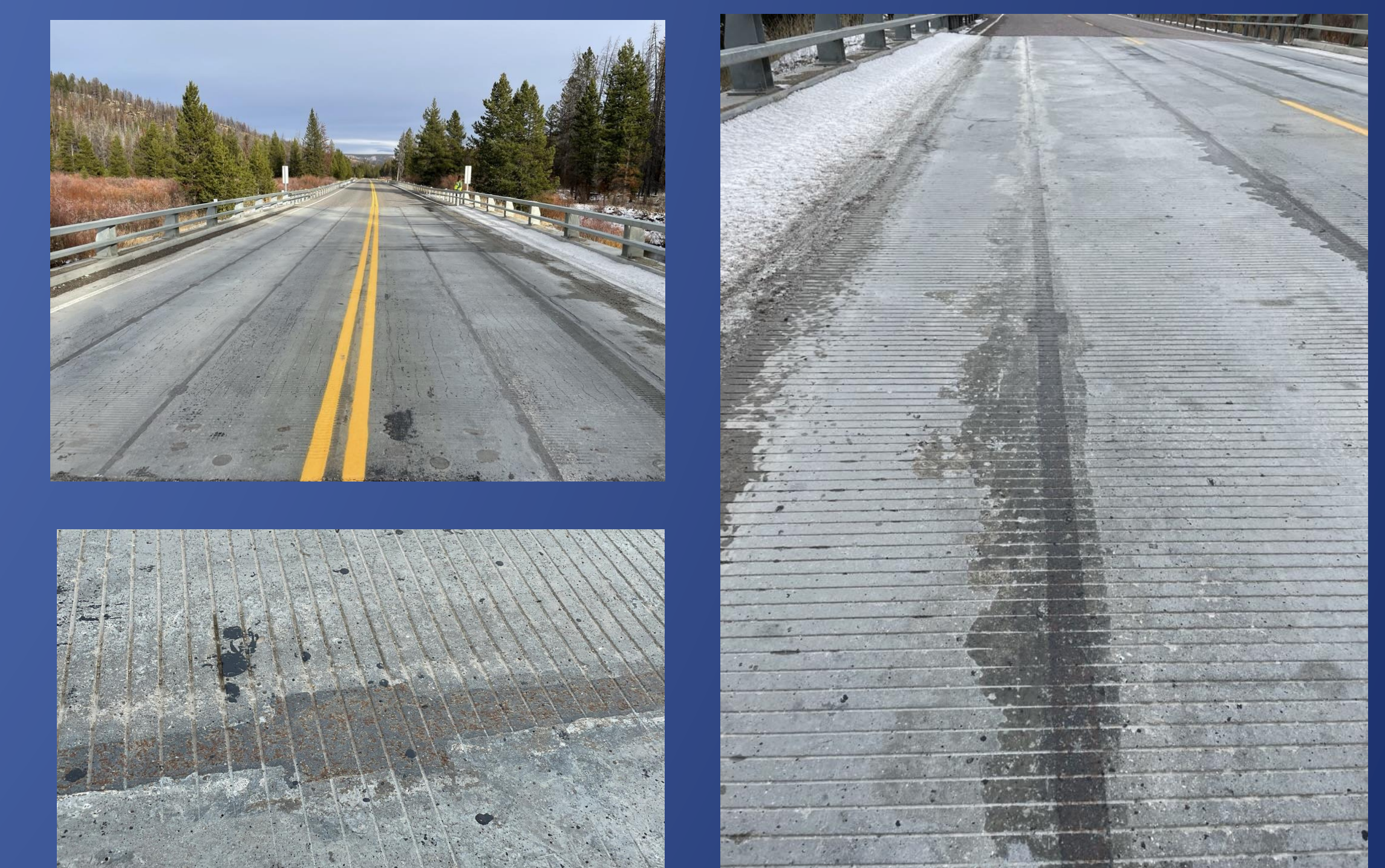
Bridge Observations at 1 Year
