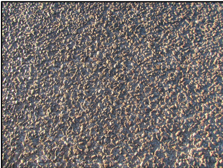
← View of current surface of PMS with chip seal on the roadway.
