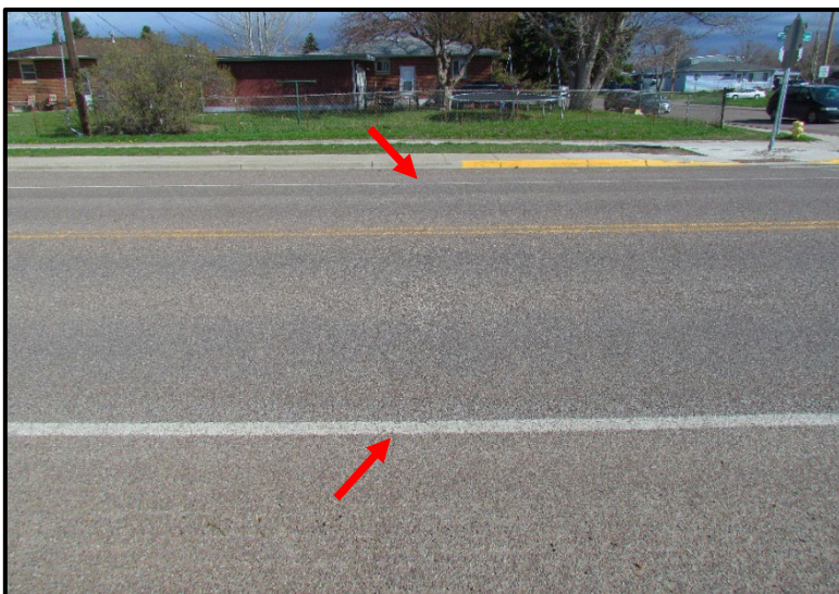
← Although difficult to see in this image; one low-severity longitudinal crack has appeared on the project near Riverview Blvd intersection (red arrows).
