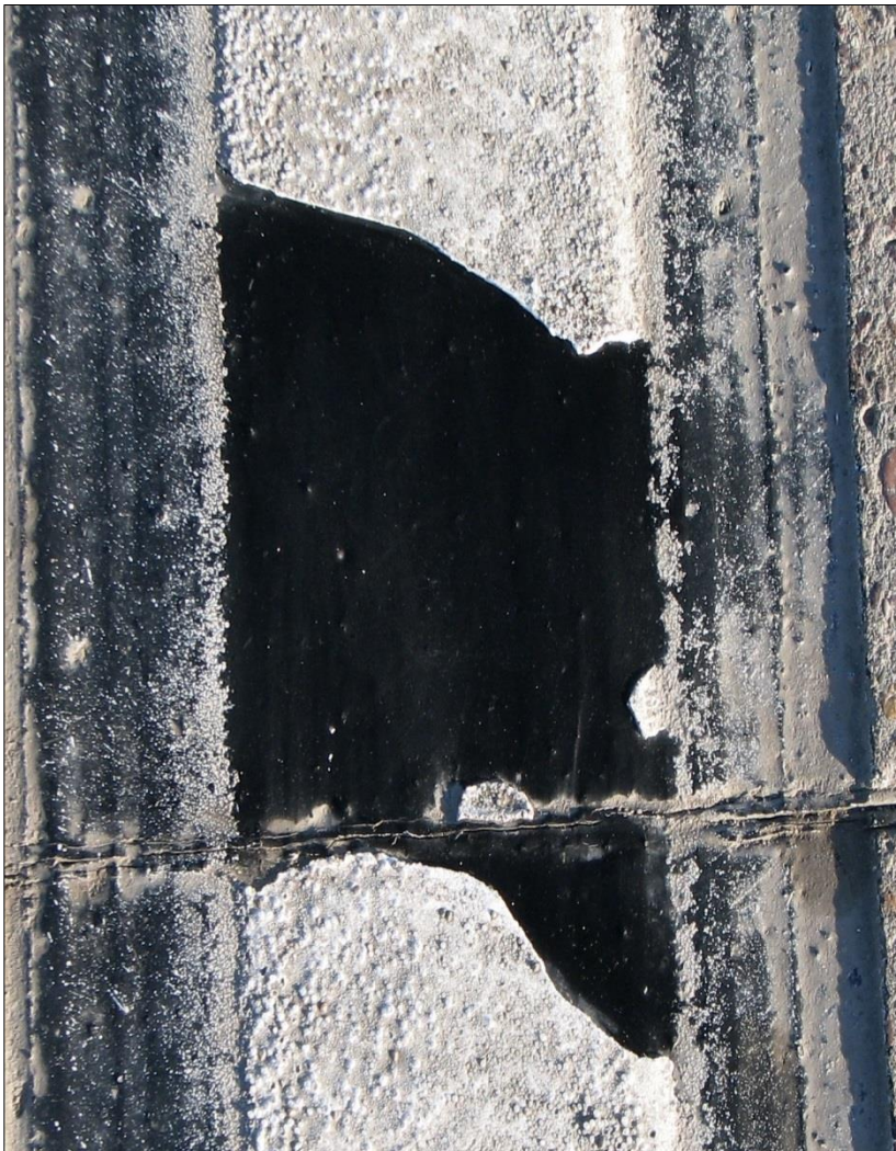
← In observing actual traffic driving over the contrast striping, this section was seen to pop off as a vehicle tire drove over it.
