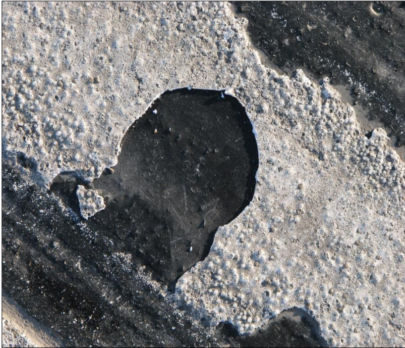
← Close up of partial white to black epoxy binder delamination.
