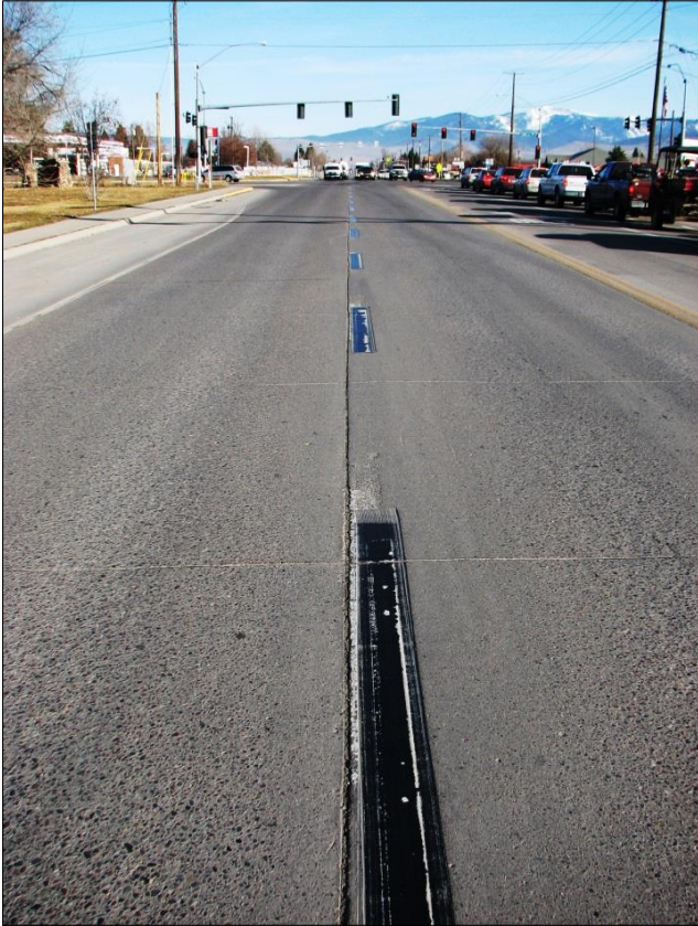
← Southbound of South St. – View North: About 14 skips lacking white stripe.
