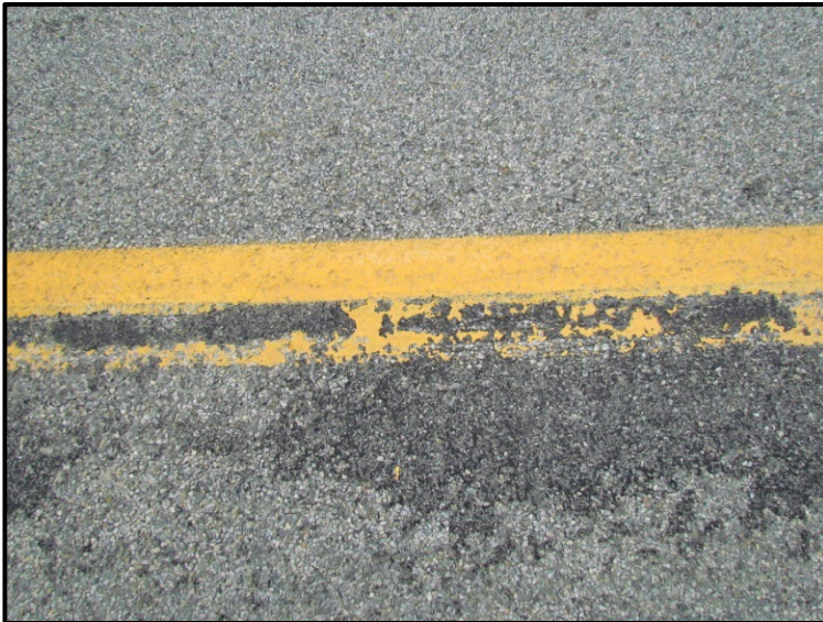
← ↓ Close up photos of the centerline without the rumble strips at varying distance at approximate RP 8.5. There was more chip stripping through the CS2 section compared to TS1.
