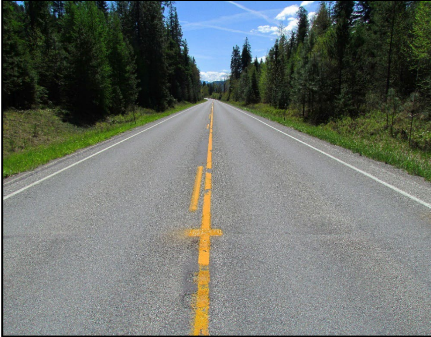
← Transition of TS1 and CS2 at approximate RP 8.2, view east. No visual distress of the CS2 longitudinal joint was observed.
