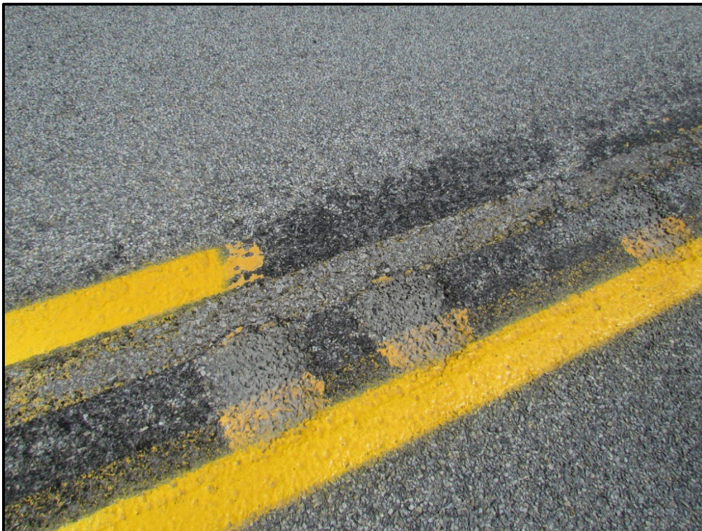
↑ RP 6.5, close-up view. Closer view of the chip stripping.
