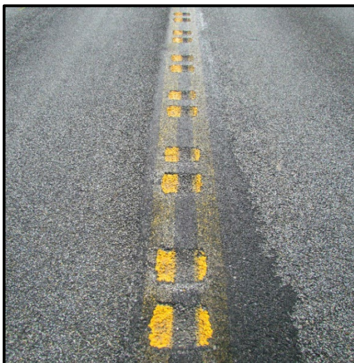
← Example of chip loss and striping damage assumed from snowplow activity.
