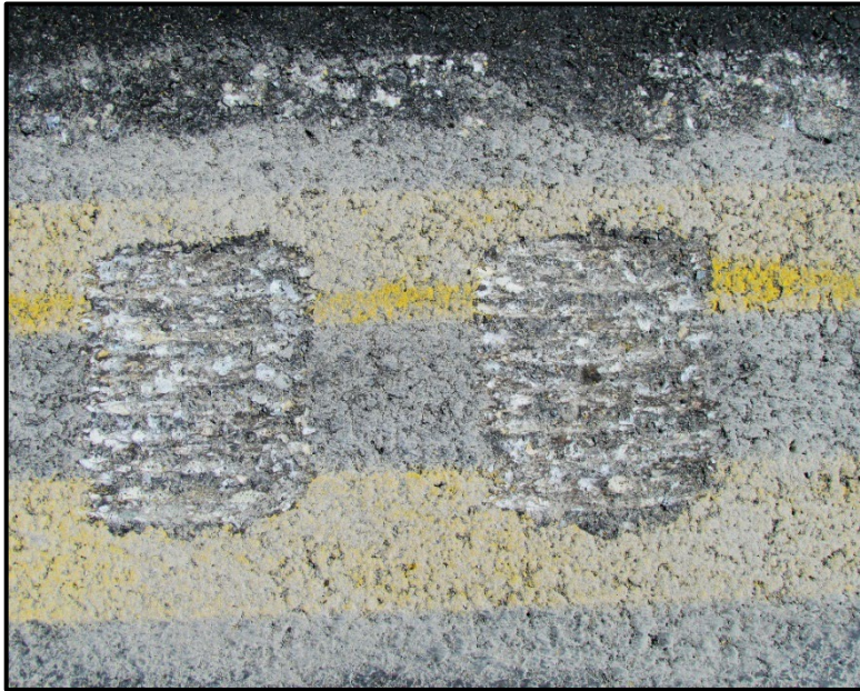
← Additional close-up of milled rumble strip in no passing zone.
