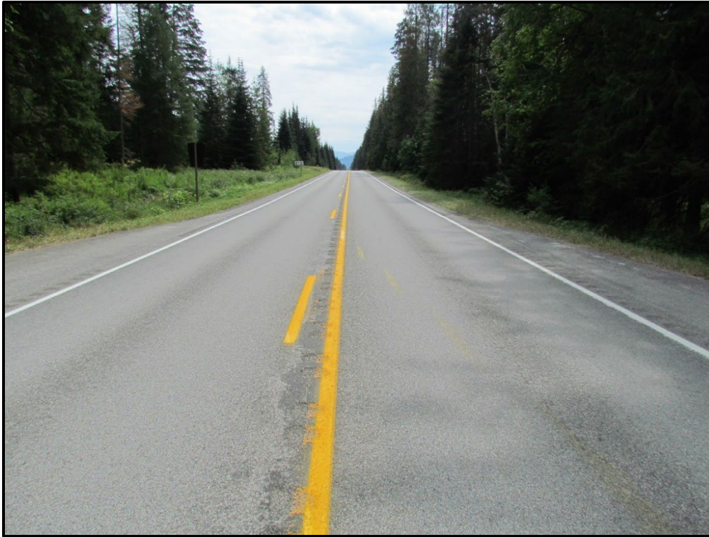
↑ RP 6.5, view east. Overview of TS1 highlighting a section of chip stripping at the centerline.
