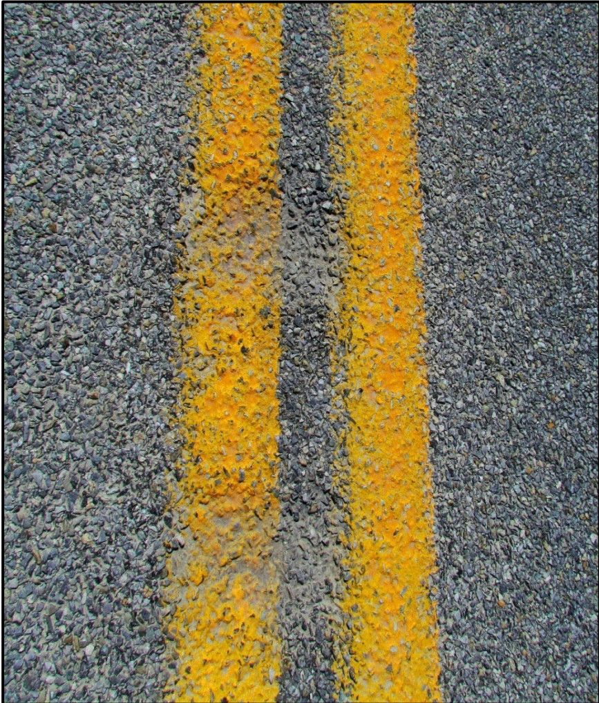
← Representative close-up of TS1 longitudinal joint at RP 5.
