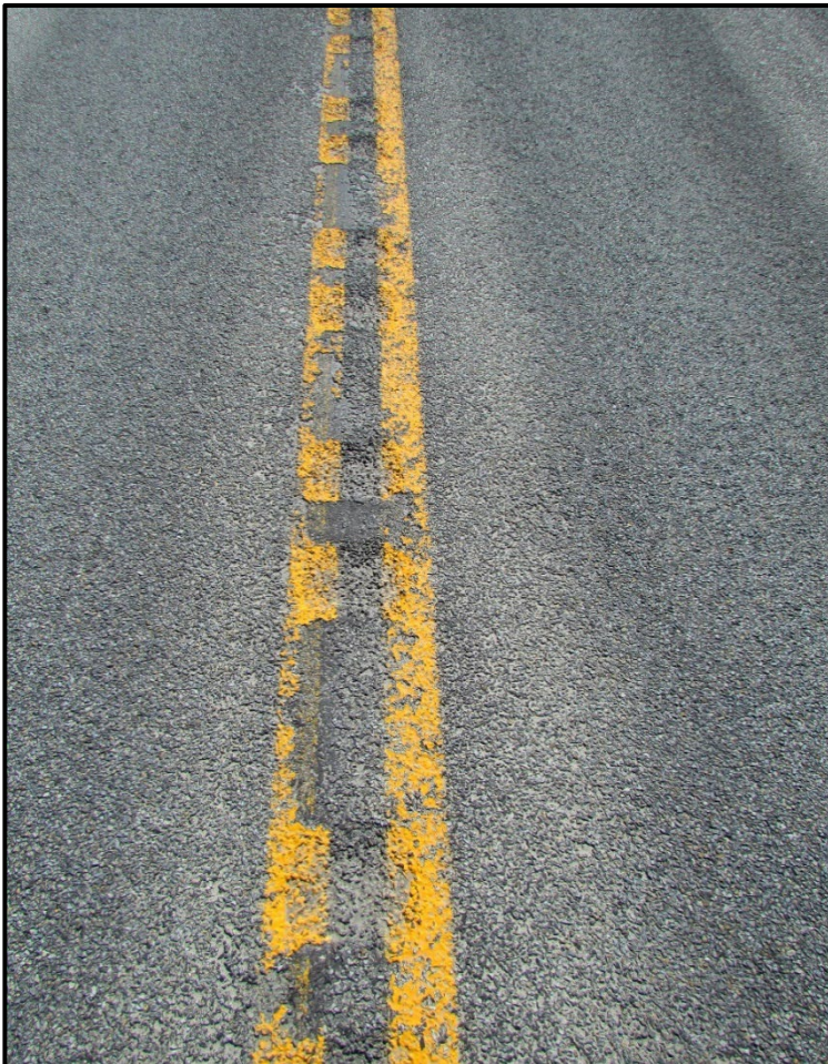
← Close-up section of CLRS. No visual distress of the TS1 paving joint was observed.
