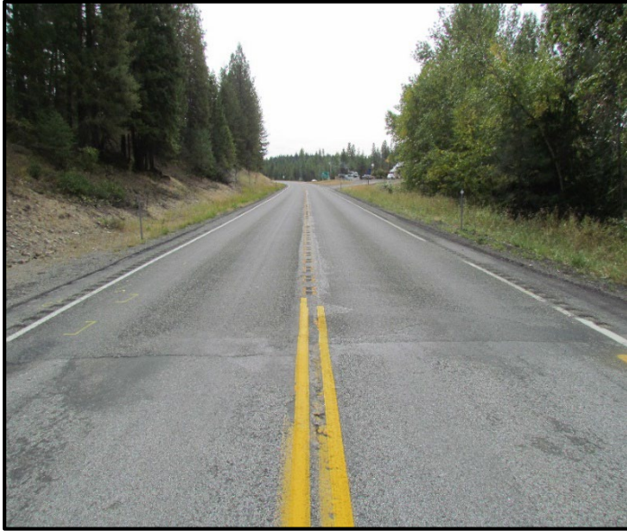
← Section TS1 at the Montana/Idaho border. The section of CLRS begins at RP 0.0, view east.
