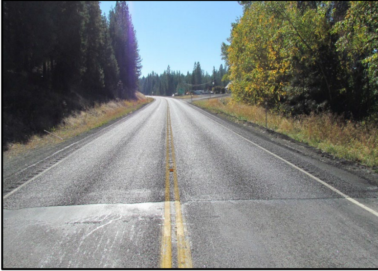
← Completed project. Roadway has received chip seal with a fog seal. View east at RP 0.0, start of TS1.
