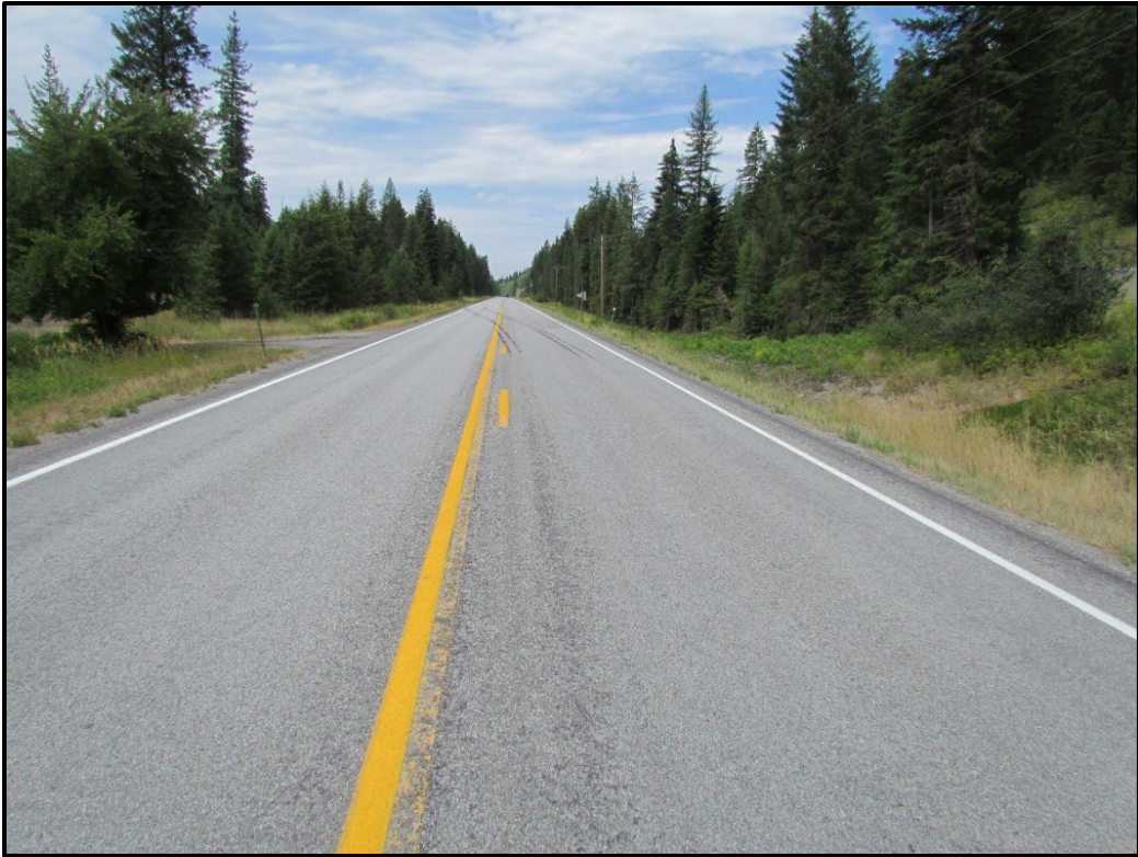
↑ RP 10.0, view west. Overview of the CS2 section highlighting an area of chip stripping.
