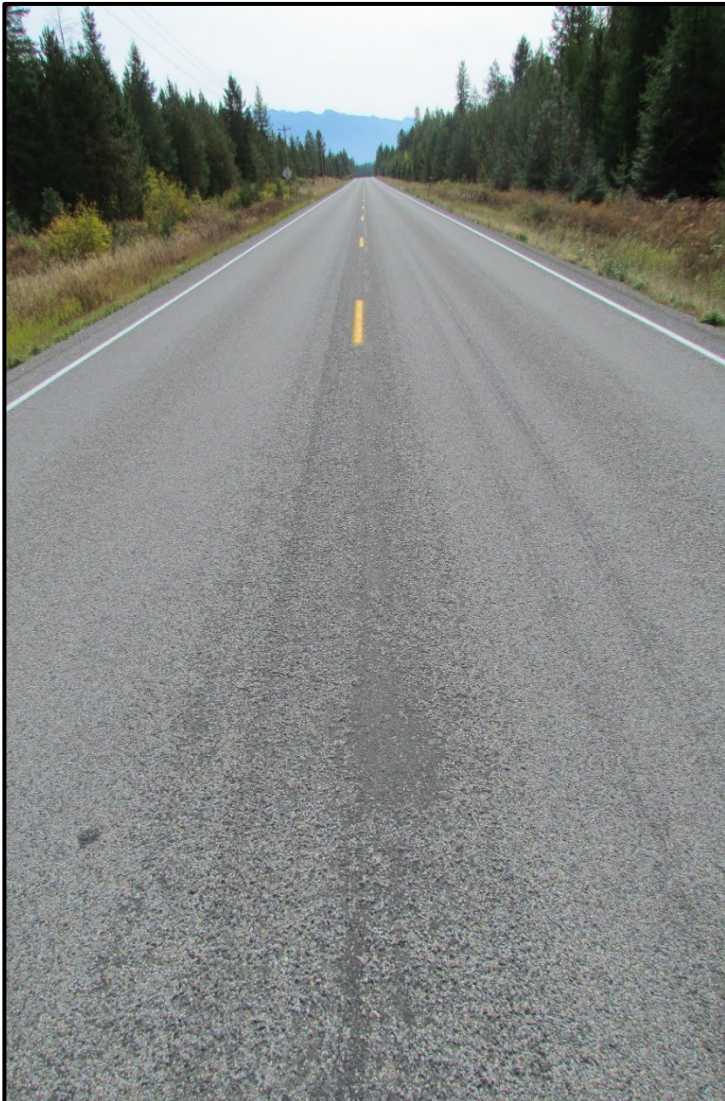
← Representative view of CS2, non-CLRS, RP 12.5, view east. No visual distress of the CS2 paving joint was observed.
