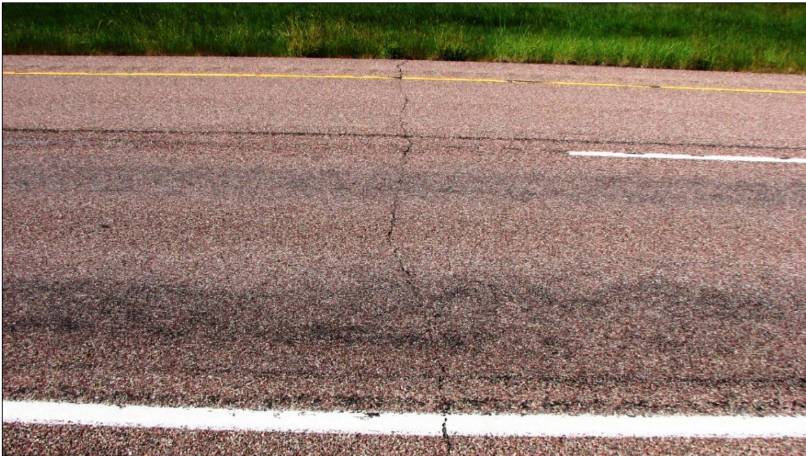
↓ Example of low-severity cracking on un-sealed south section (2011)
