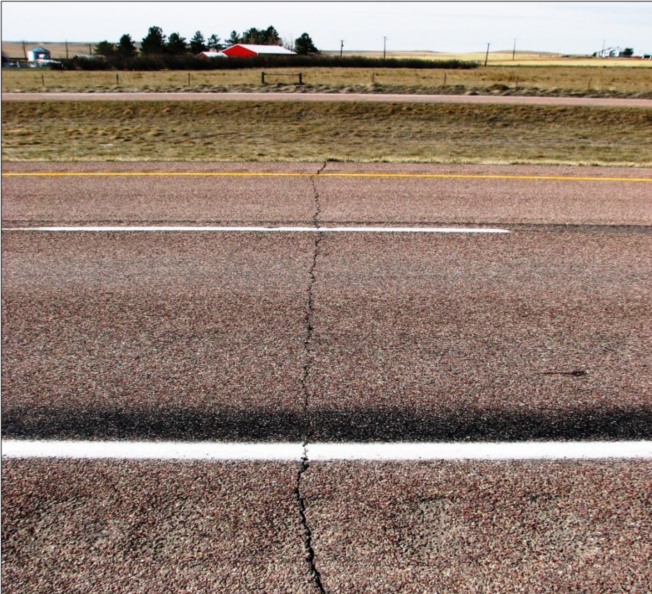
← Example of low-severity cracking on un-sealed south section (2013)
