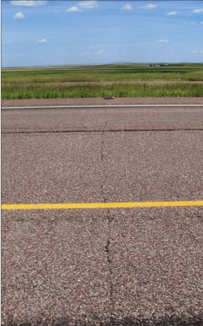
← Example of low-severity cracking on sealed north section (2009)
