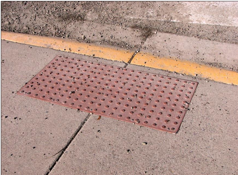
← General example of stainless steel DWD still in service.
