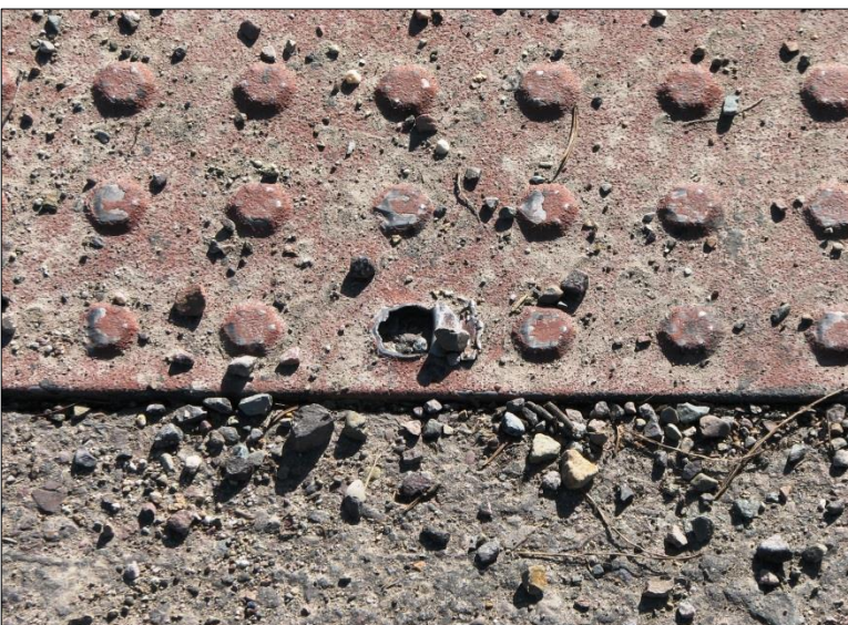
← Example of the type of distress seen on this project with stainless steel DWD apparently caused by snow plow maintenance.
