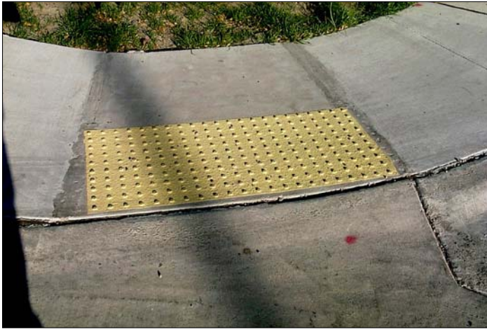
Installation 5A: located at northwest intersection of 1 st Ave. N. W. and 6 th St. N. W.
