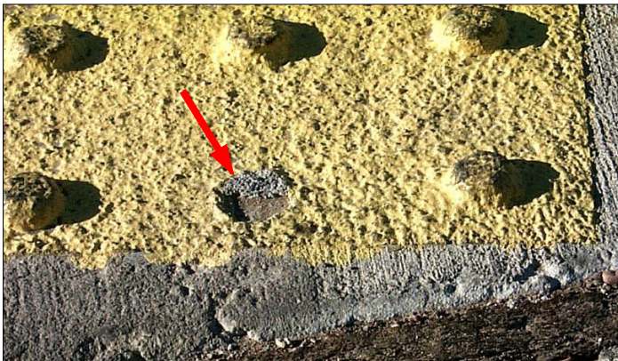
Installation 5B: Close-up of missing dome. It is unclear how this dome was lost; however there was evidence of heavy-lugged tire treads on top and around the mat. You can see the skid tracks on the top surface of the domes.
