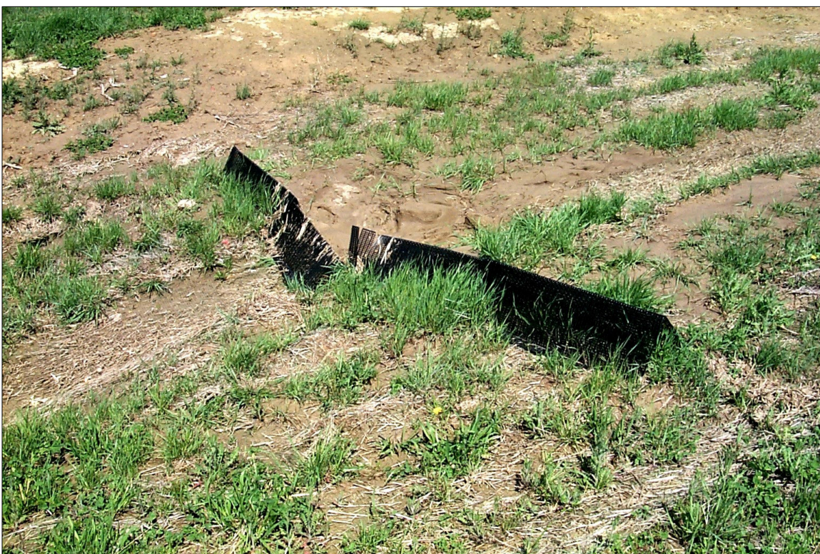
June 2007: Above image shows break in the PPB section either due to improper installation or a significant hydraulic event. However the device appears to be functioning nominally.
