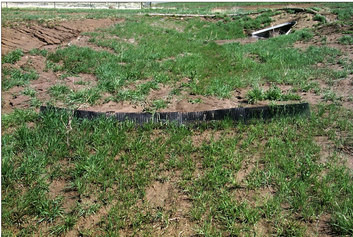
June 2007: Same image as previous with the view of the PPB from the downstream side.
