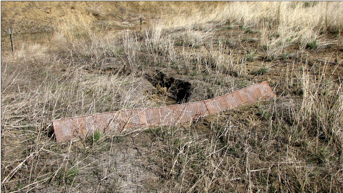
May 2008: PPB used to mitigate further erosion of slope. An erosion blanket was placed directly upstream of the device; however it is difficult to see in this image.
