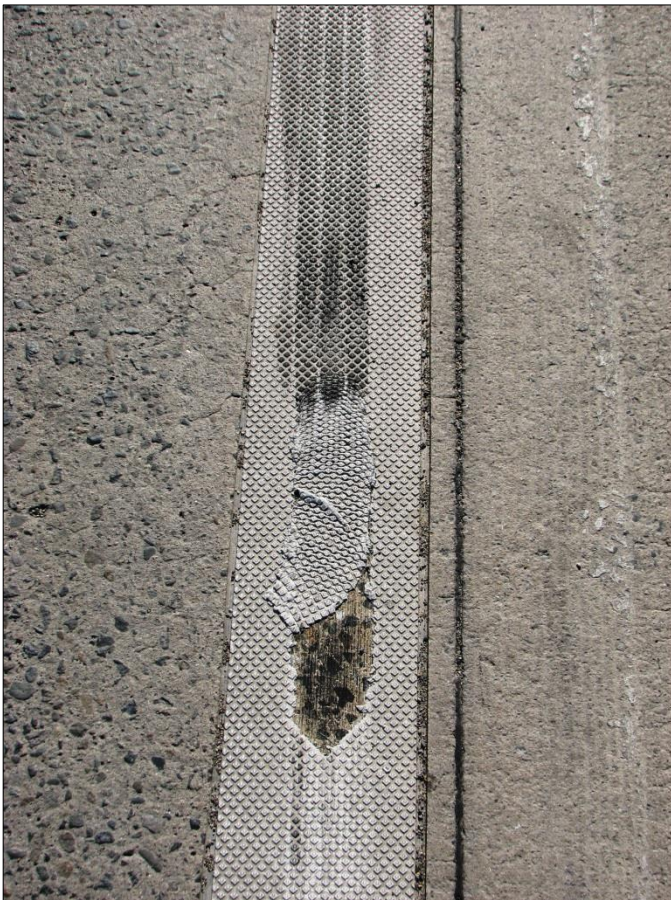
← Damaged caused by sudden braking by a vehicle is apparent in this image.
