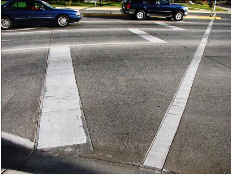
↙ More examples of the type of tape distress with the 3M Stamark project.
