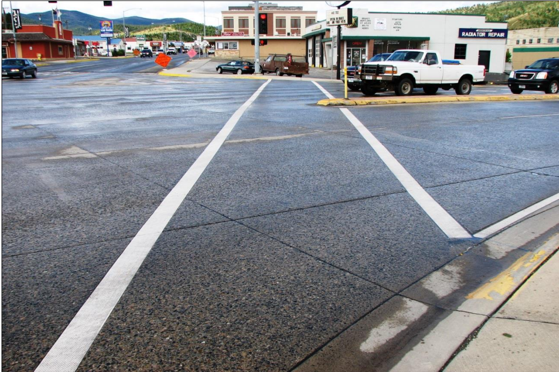
↑ Image of West Lyndale: westbound, west side pedestrian lines shortly after installation.
