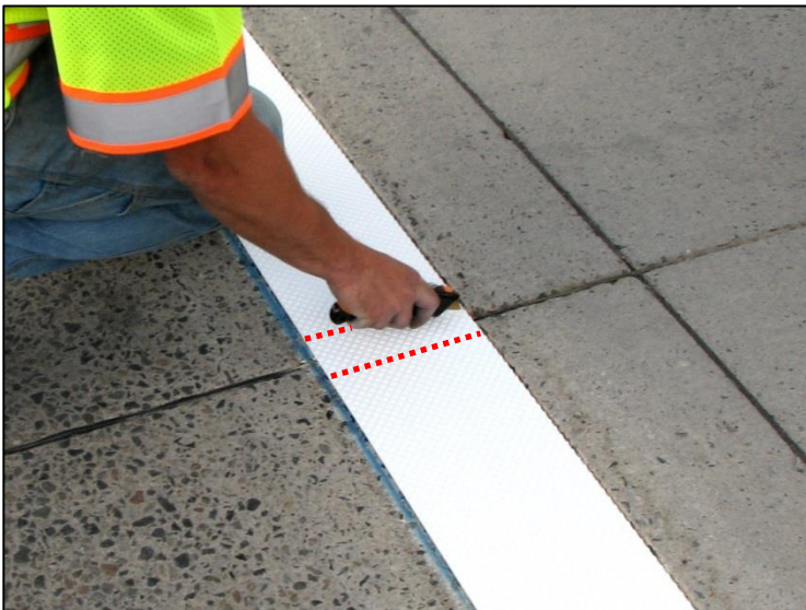
← Those markings positioned over pavement joints are cut roughly 1" on either side of the joint (red dash lines).
