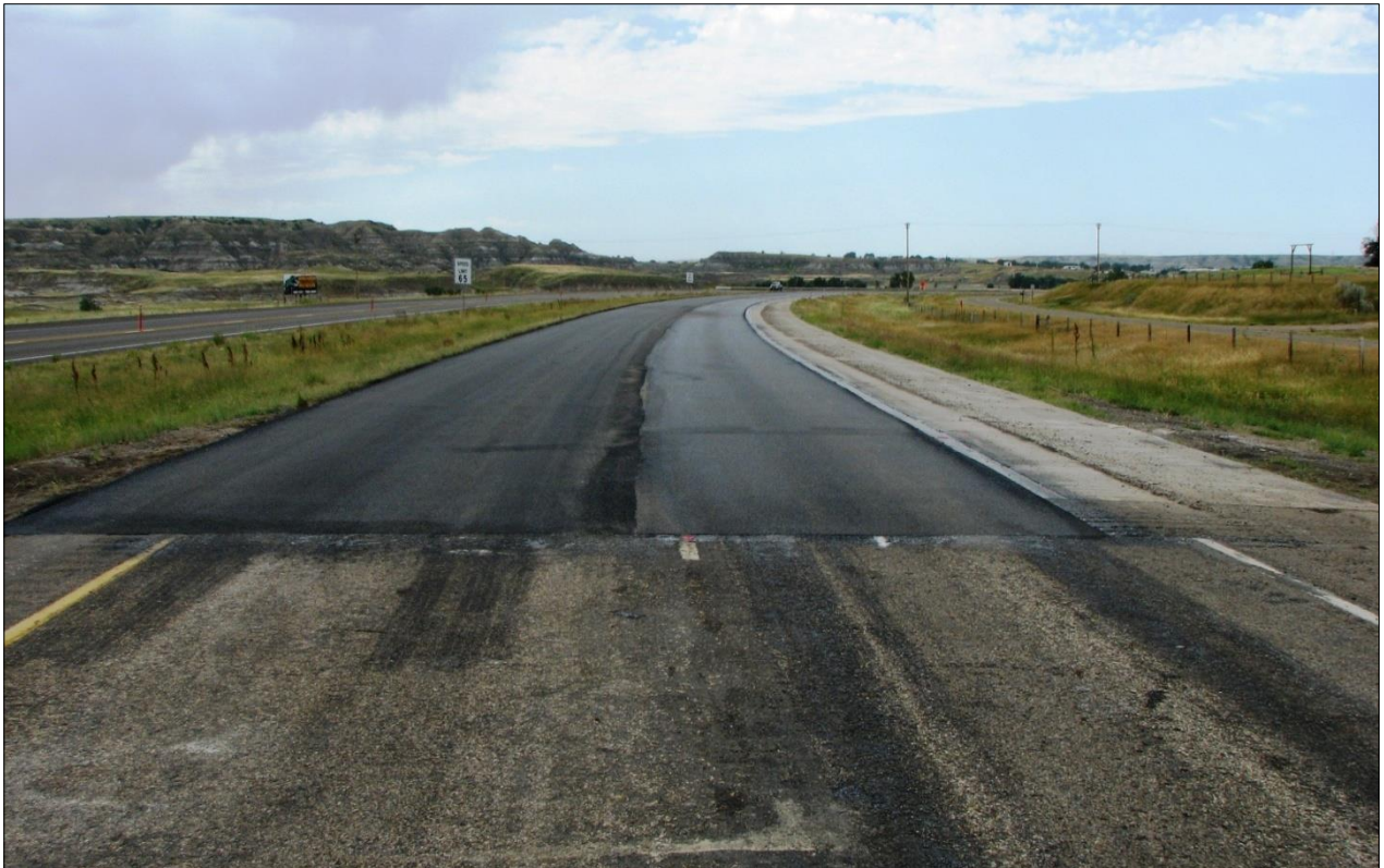
↓ Completed paving of the travel, shoulder and passing westbound lanes at start of east end of project.
