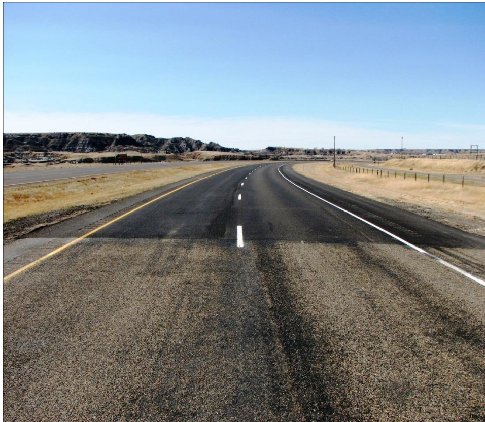
← Westbound PMS lanes at east end of project. View is looking west.
