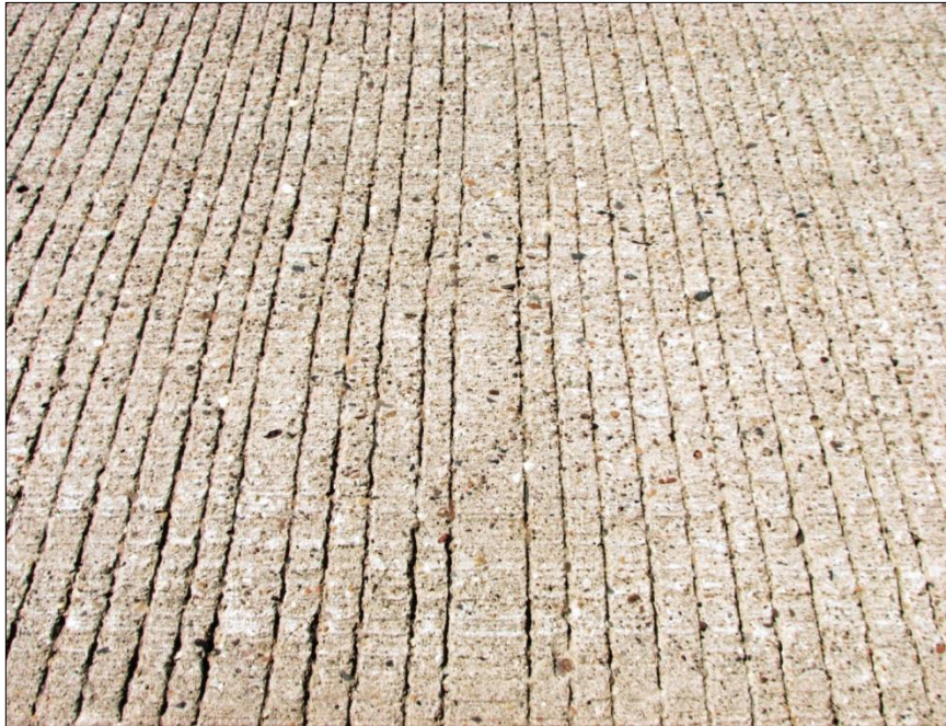
← Condition of PCCP prior to diamond grind
