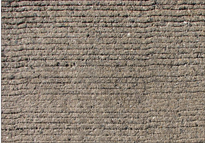
← Surface textures in both lanes appeared to be in good condition since installation.
