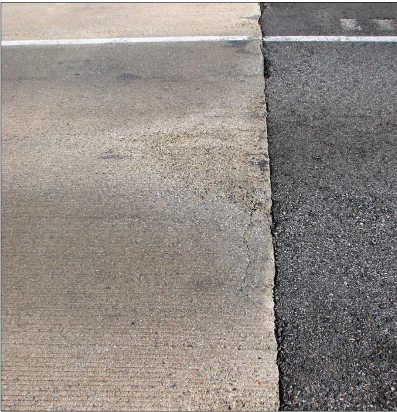
← Closer view of the plow scrapes on the PPC travel lane in addition to some localized stress cracking near the joint approach (red arrow).
