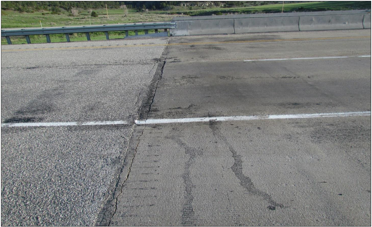
↓ East bound-East end transition joint of deck to pavement; transverse cracking apparent on the PPC which runs along the entire east span.
