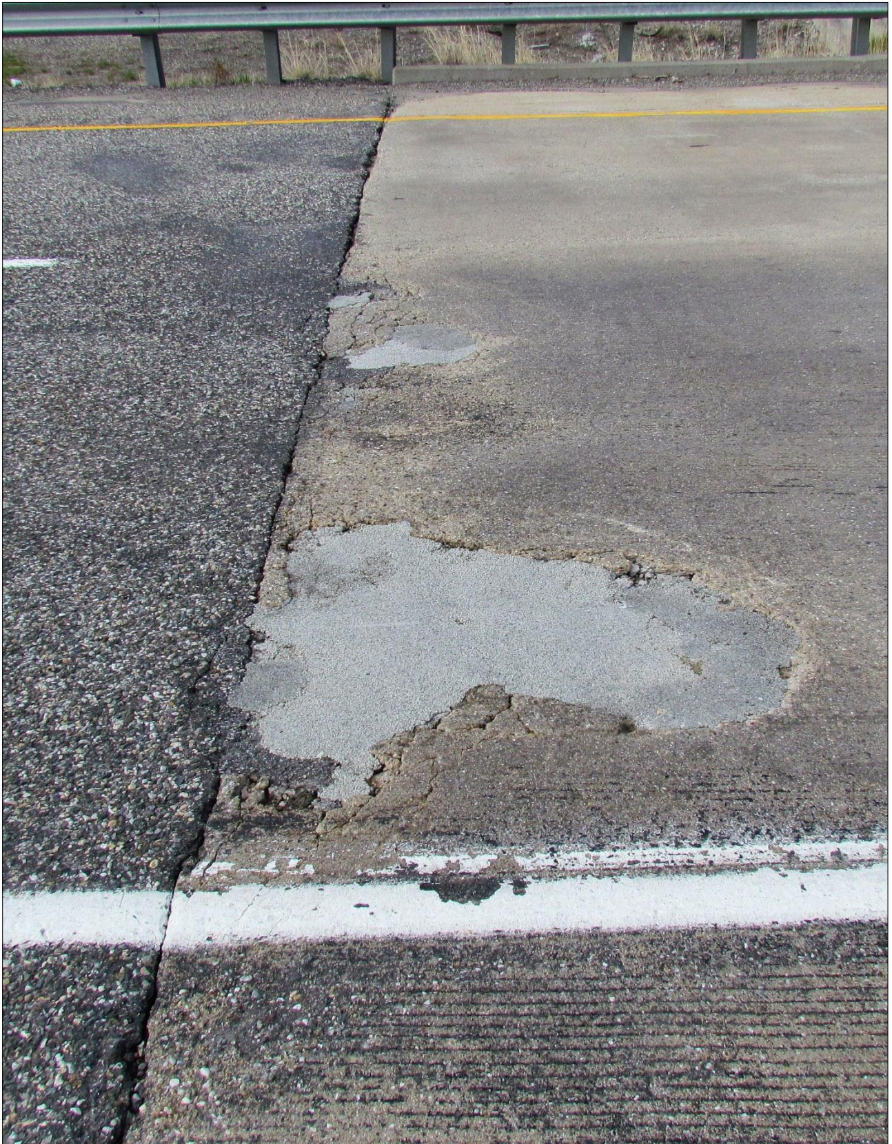
↑ Additional view of deck patching at east end of westbound deck; continued spalling is apparent.
