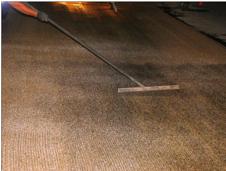
← Longitudinal tining is reapplied for mechanical texture as one of the last steps in completing the PPC run.
