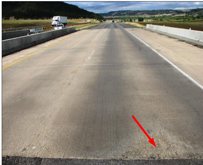
← Surface textures in both lanes appeared to be in good condition after the first year since installation.
