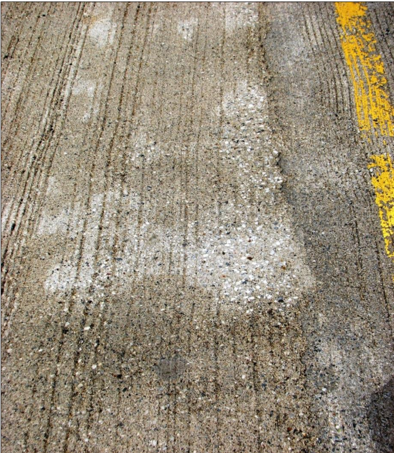
← Close-up of PPC abrasion by plow passes (south deck shoulder).
