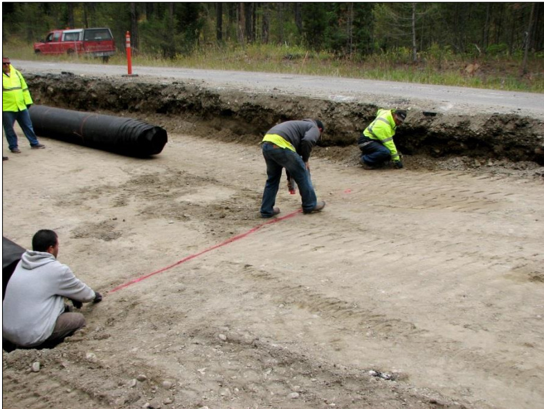
← The contractor applied a paint line to mark the starting edge of the first section of SSDL.
