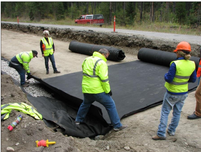
← The SSDL is rolled out and the leading edge is placed directly over the edge drain.
