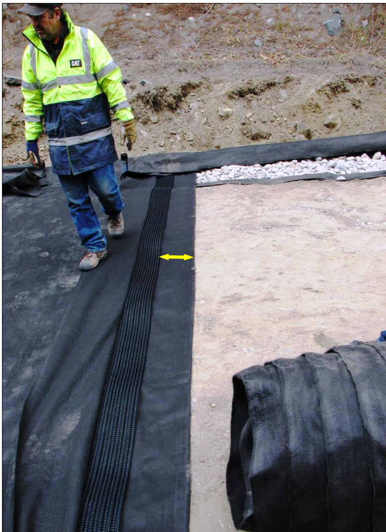
← The fabric filters (top and bottom) are set wider than the drainage core to ensure ample length for an effective overlap seaming of the subsequent adjacent rolls (yellow arrow).
