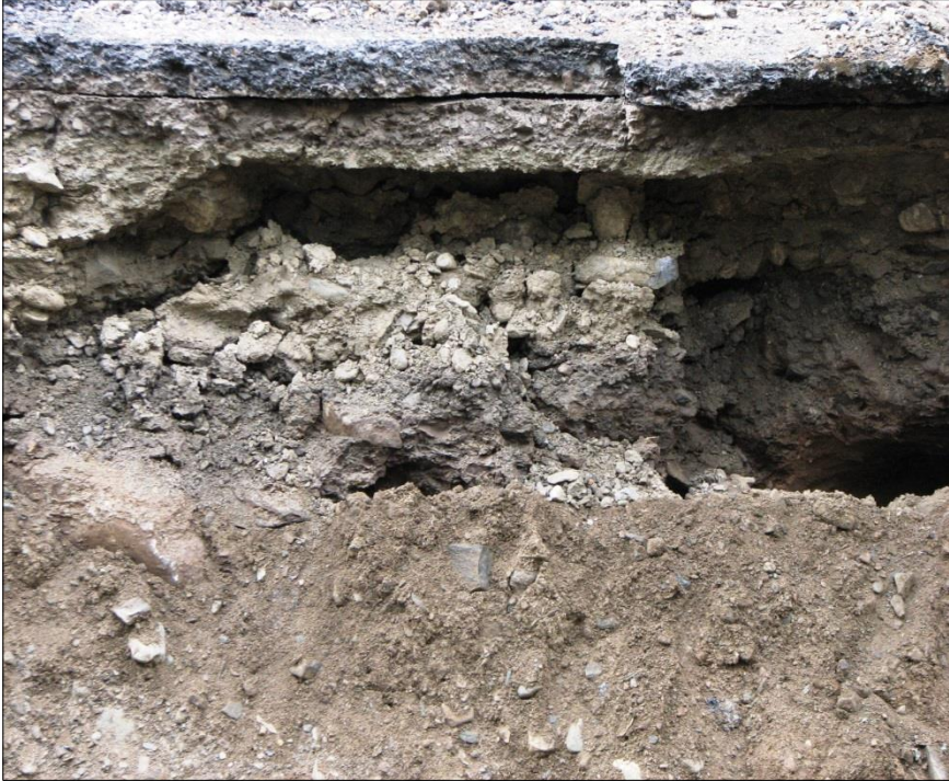
↙↘ Southbound excavated cross-section of roadbed; two photo examples of the previous repair constructed several years ago.
