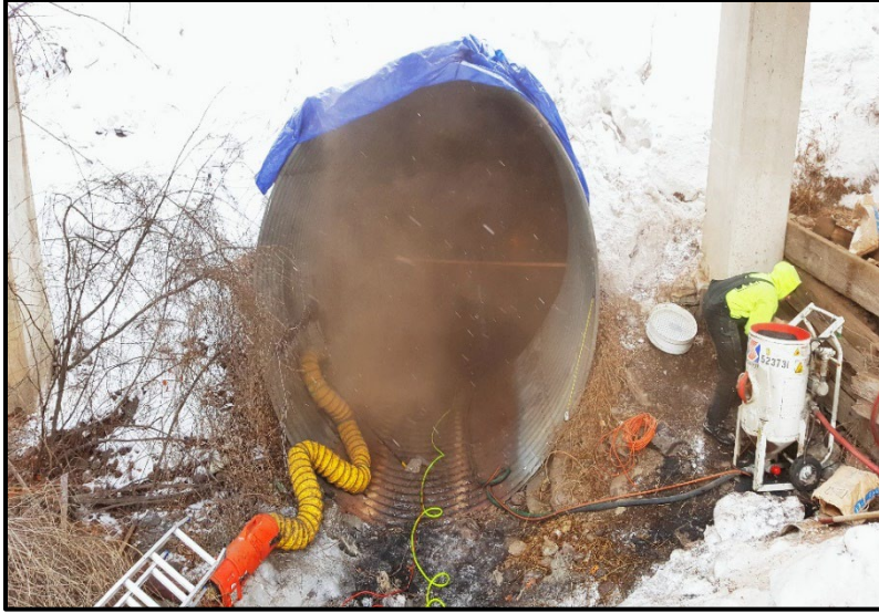
↙ The base of the culvert where corrosion took place is sand blasted (Kleen Blast Abrasives) to bare metal and vacuumed clean.
