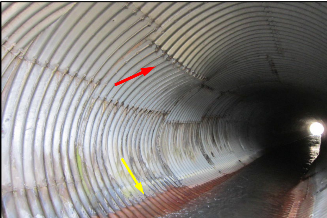
↑ Representative image of the observed sagging in the top panels of the steel plate arch culvert. Deflection estimated at six inches inspected in 2014 (red). Corrosion also apparent at the base of the culvert (yellow).
