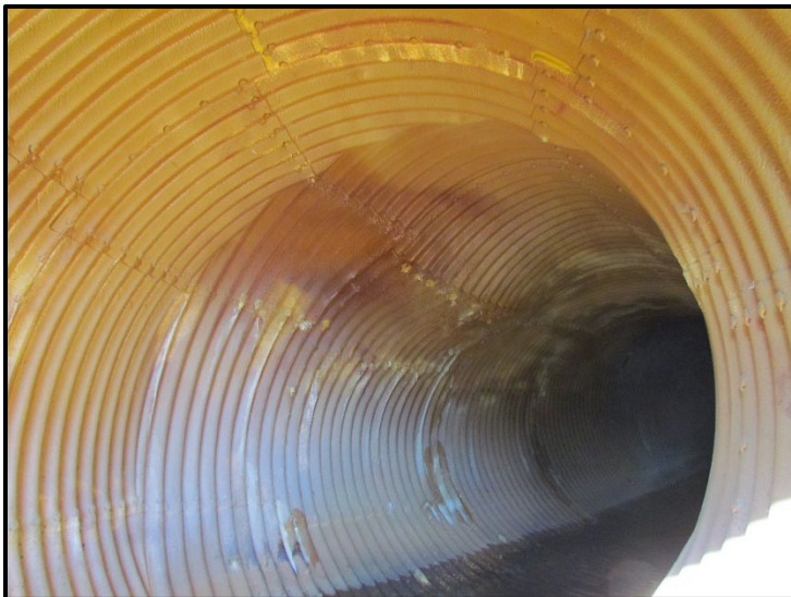
← View highlighting the original deflected section of the culvert. There's no sign of failed adhesion or SprayWall liner separation from the culvert.
