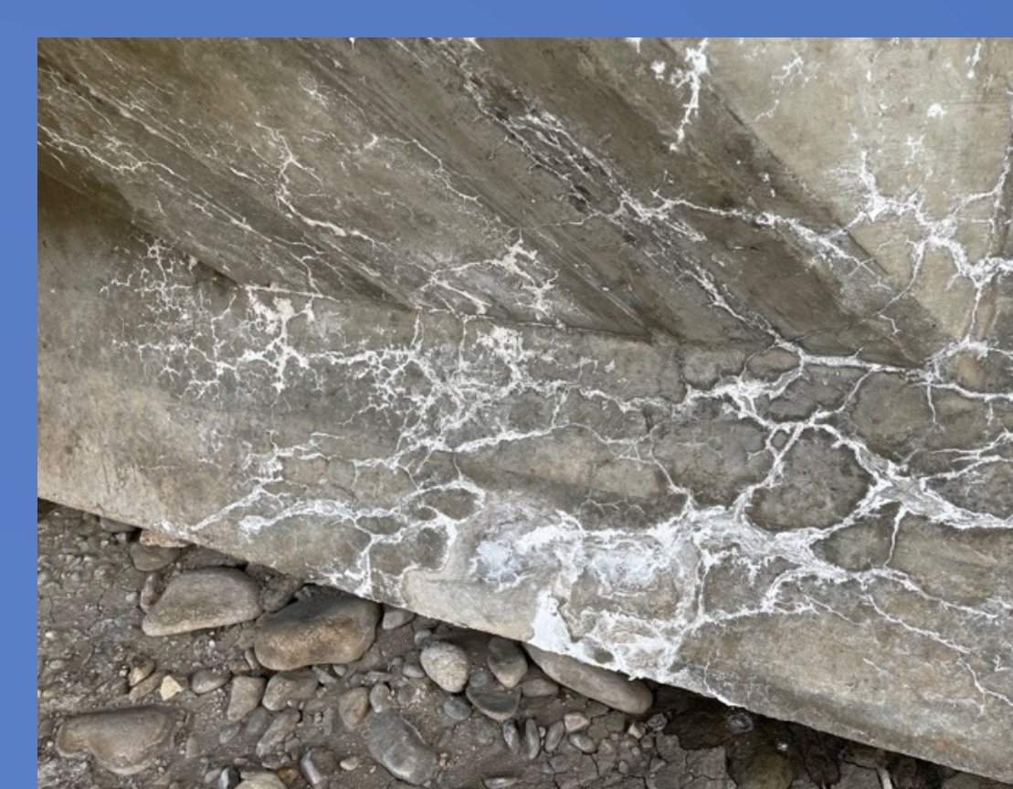
Backwall and Beam Showing Signs of Distress
