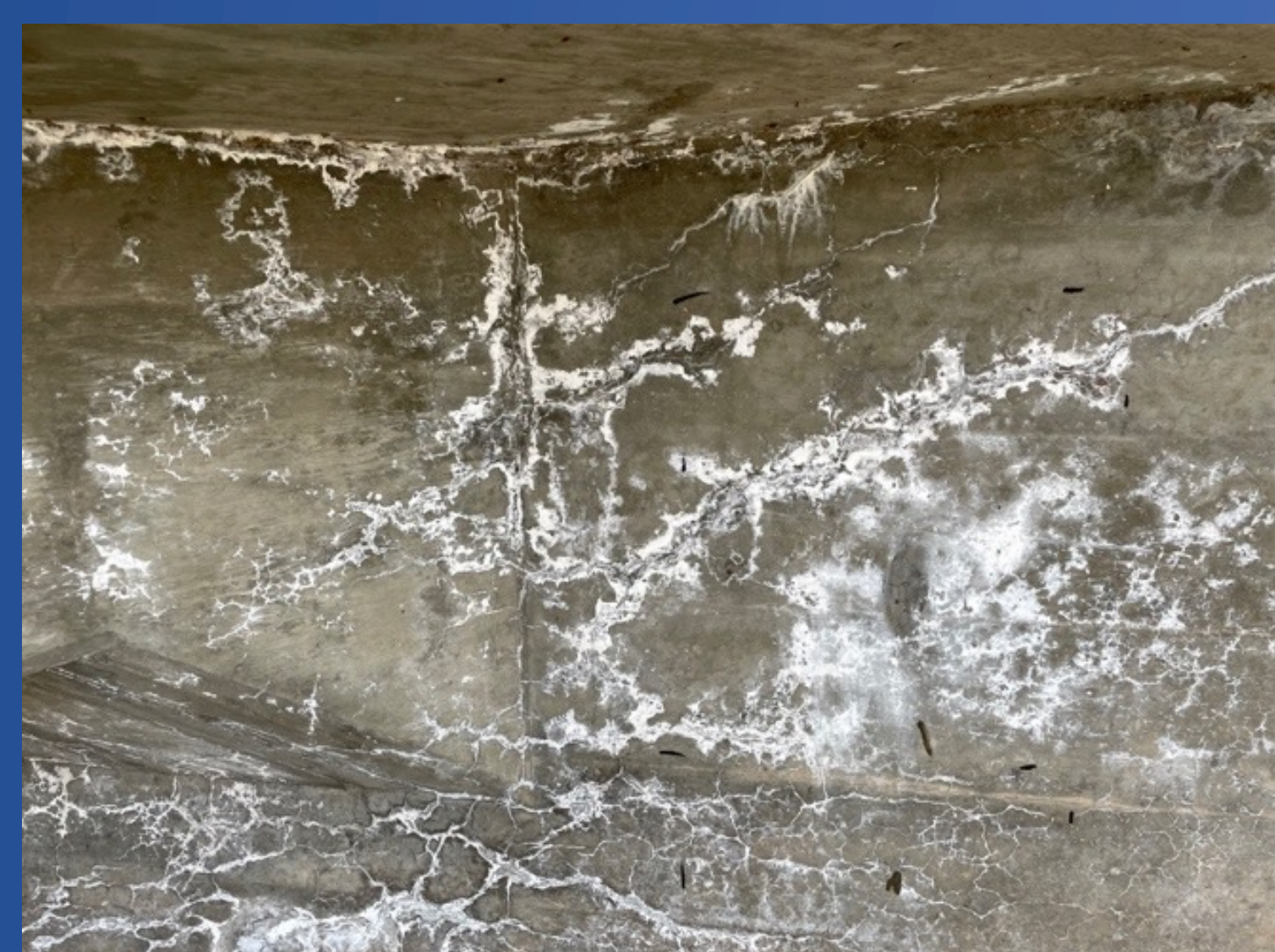
Typical ASR Crack Patterns
