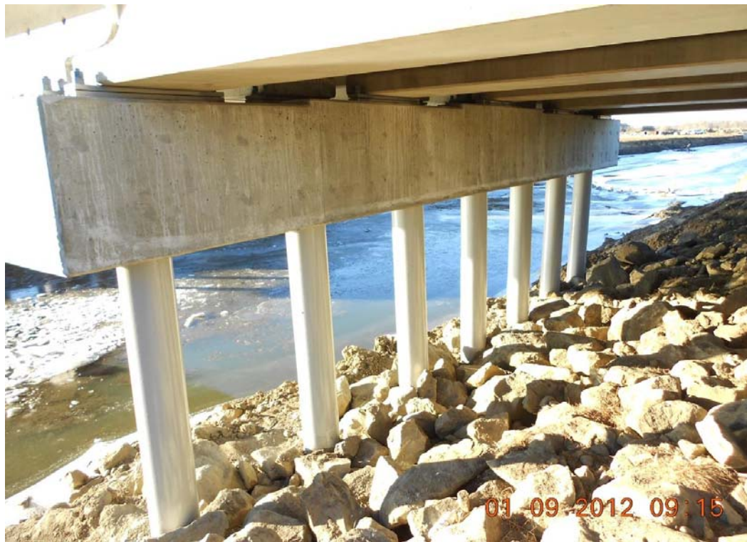
Figure 1. Typical concrete-filled steel pile and concrete pile cap bridge substructure support system (Kappes, 2012)
