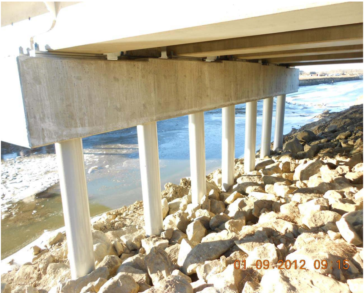
Figure 1: Typical MDT concrete-filled steel pile and concrete pile cap bridge substructure support system (Pryor Creek Bridge near Huntley, MT - courtesy of MDT (2012))
