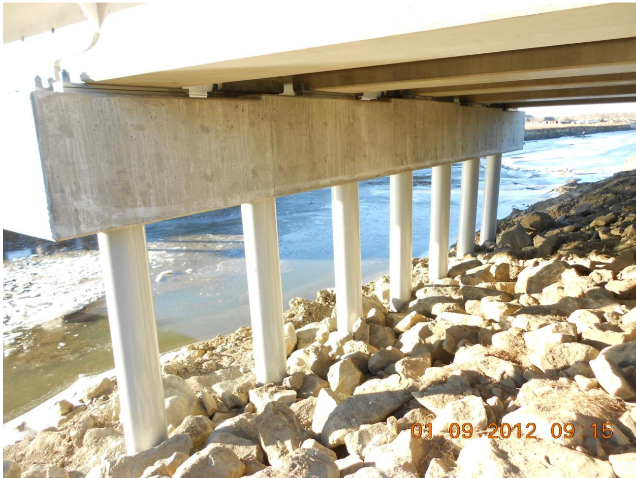
Figure 1: Typical MDT concrete-filled steel pile and concrete pile cap bridge substructure support system (Pryor Creek Bridge near Huntley, MT - courtesy of MDT (2012))
