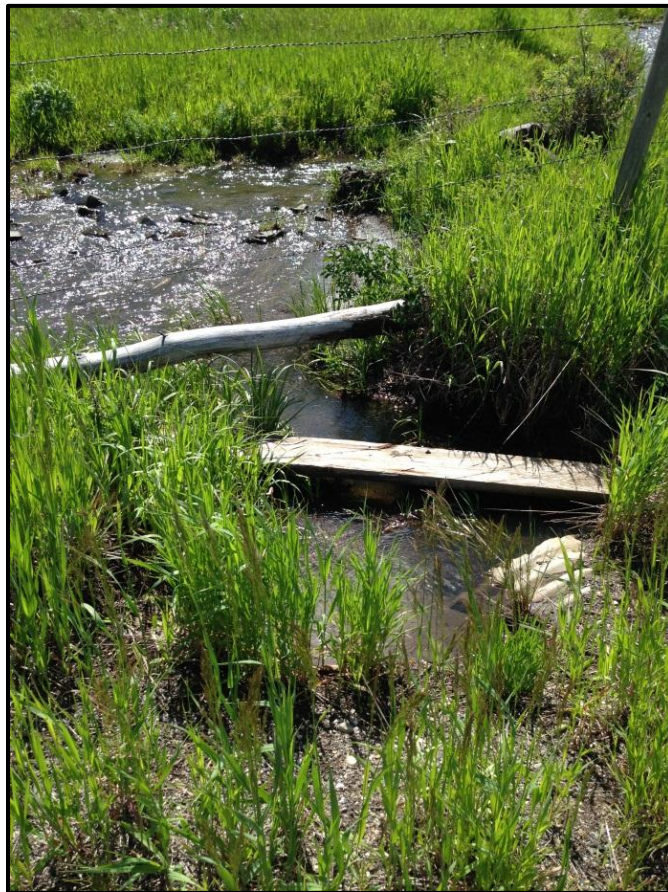
Photo 76. Looking at a plugged culvert on an unnamed tributary to Cache Creek. RP 24.7.
