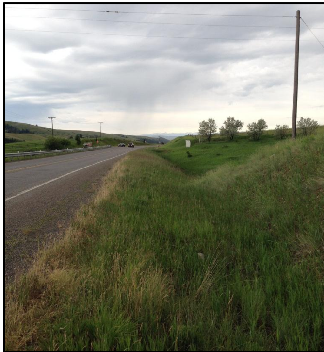
Photo 40. Looking at unprotected substandard cut/fill slopes along MT 86. RP 4.1.
