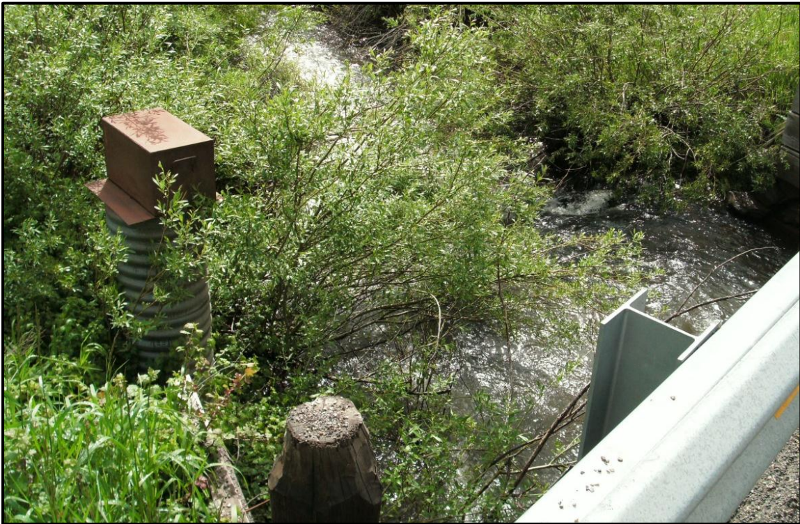
Photo 21. Looking downstream (southeast) where MT 86 crosses the Middle Fork Brackett Creek. Also pictured is a stream gauging station on the left bank. RP 19.9.
