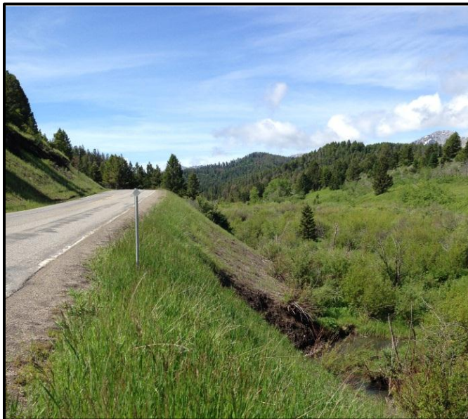
Photo 74. Looking at unprotected substandard fill slopes and substandard back slopes on MT 86 due to embankment erosion on Cache Creek. RP 22.7.
