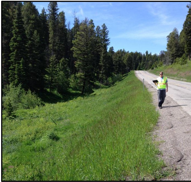
Photo 73. Looking at unprotected substandard fill slopes and substandard back slopes along MT 86. RP 21.0.
