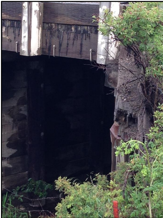
Photo 58. Looking at a damaged wing wall on a MT 86 bridge crossing an unnamed tributary to Bridger Creek. RP 9.5.
