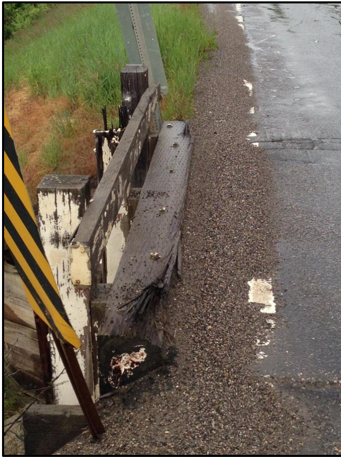
Photo 59. Looking at a damaged abutment on a MT 86 bridge crossing an unnamed tributary to Bridger Creek. RP 9.5.
