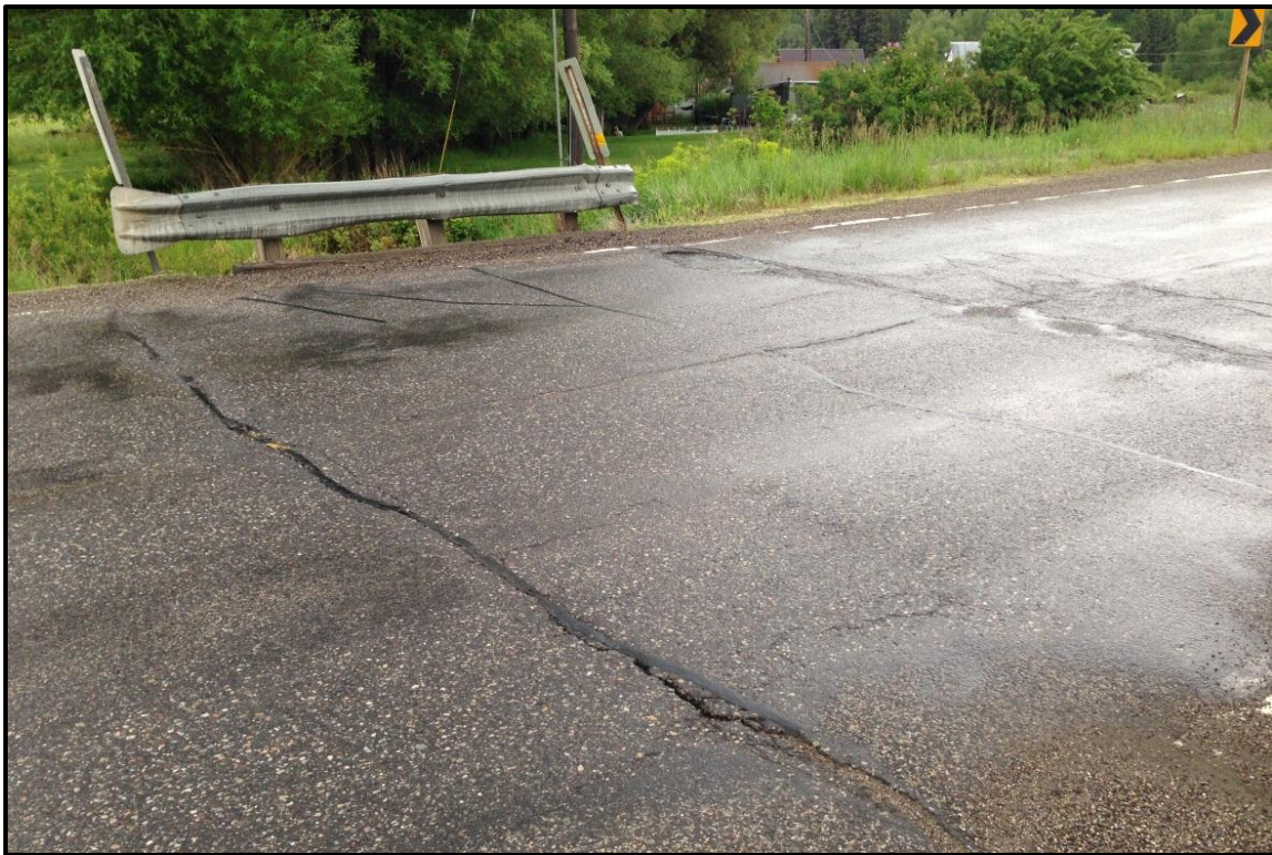
Photo 52. Looking at pavement deterioration at MT 86 bridge crossing Place Creek. RP 6.8.
