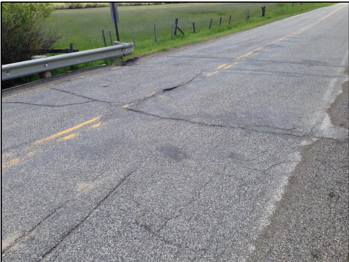
Photo 84. Looking at pavement deterioration at a bridge crossing Carrol Creek. RP 27.1.
