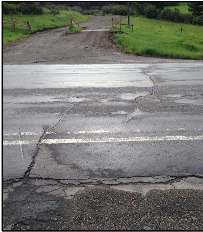
Photo 63. Looking at pavement deterioration on MT 86. RP 14.3.
