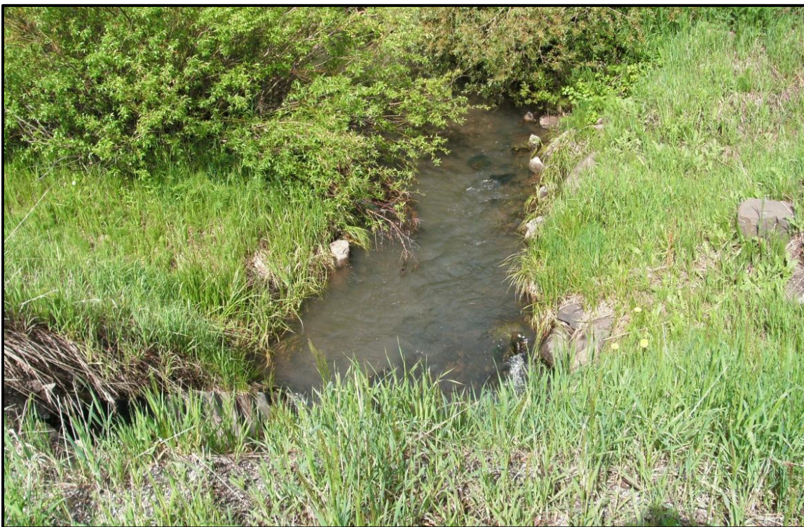
Photo 20. Looking downstream (east) where MT 86 crosses the South Fork Brackett Creek. RP 19.9.
