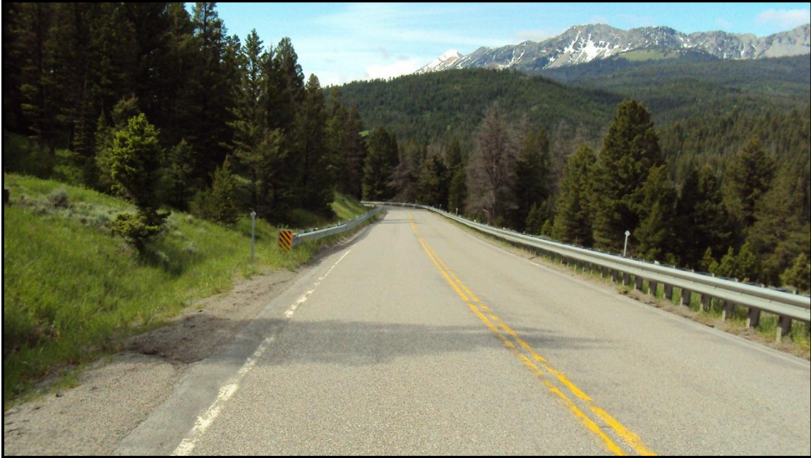
Photo 61. Looking south on MT 86, guardrail runs adjacent to the highway narrowing the traveled way. RP 13.7.
