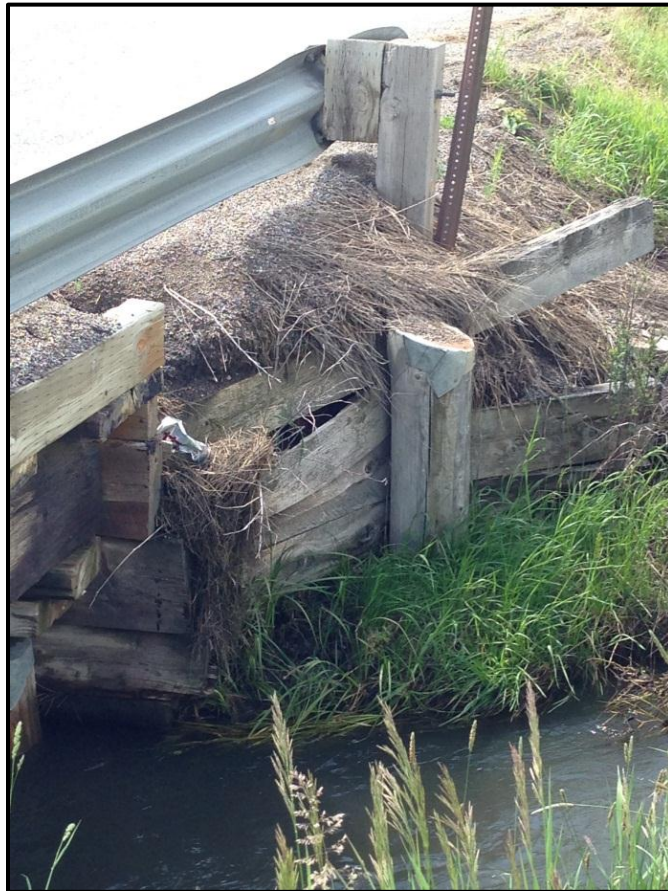
Photo 85. Looking at a damaged bridge crossing Carrol Creek. RP 27.1.
