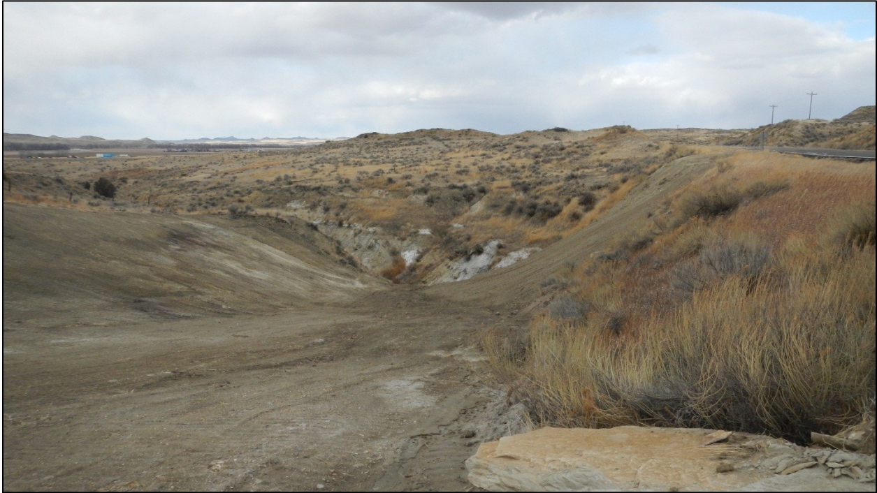
PHOTO 9: RP 4.5 LOOKING NORTH – RECENT SLIDE AREA
