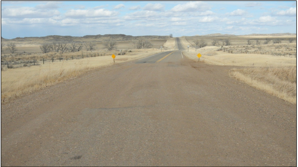
PHOTO 24: RP 17.7 LOOKING NORTH - END OF PAVEMENT
