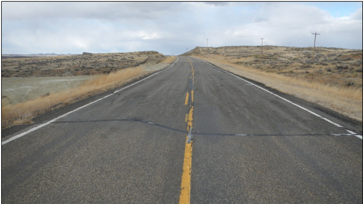
PHOTO 8: RP 4.2 LOOKING NORTH – RECENT SLIDE AREA
