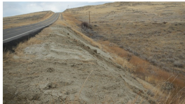
Example of slide area - note abrupt pavement edge
