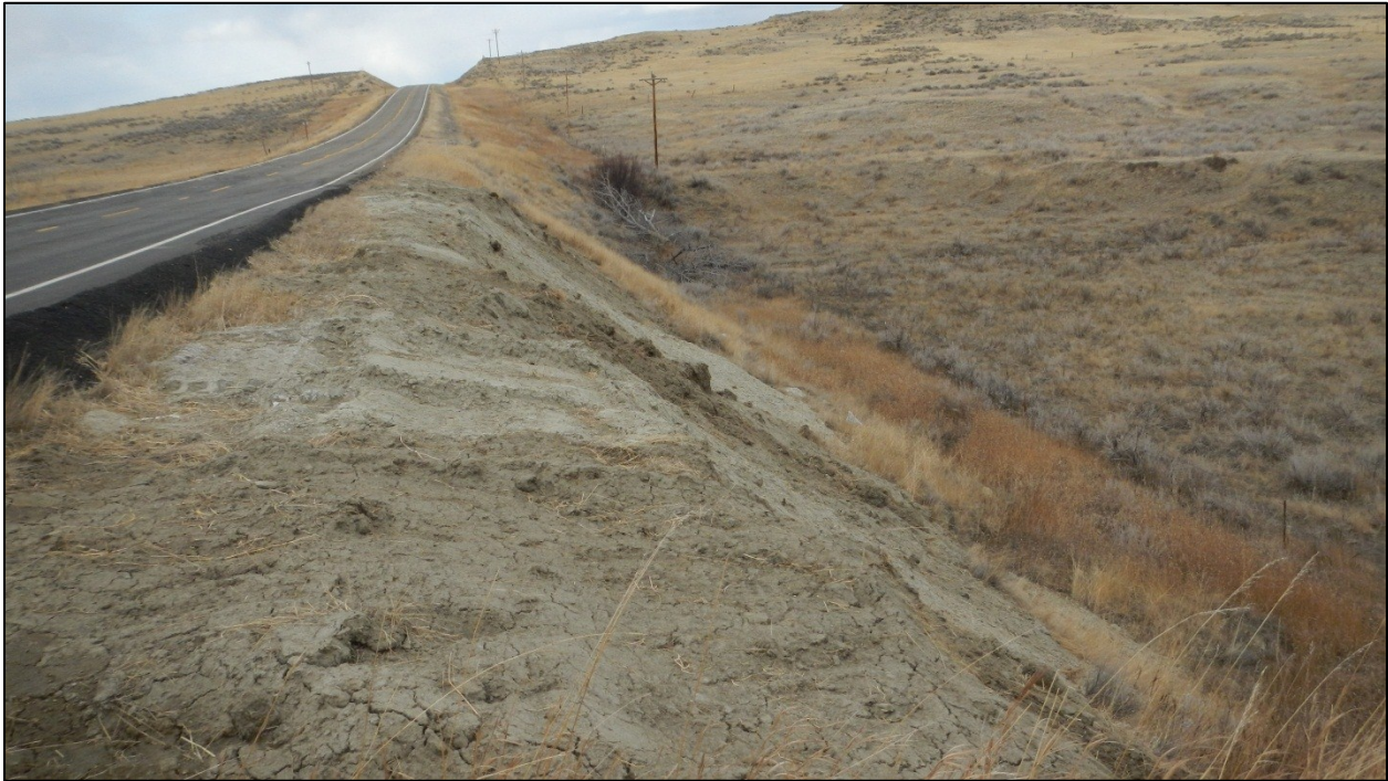
PHOTO 6: RP 3.7 LOOKING NORTH – RECENT SLIDE AREA
