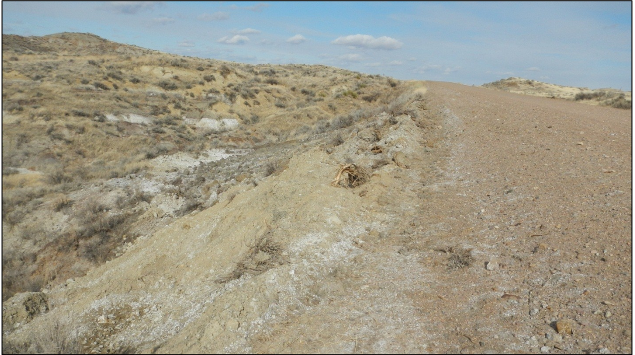
PHOTO 37: RP 27.9 LOOKING NORTHEAST - RECENT SLIDE AREA
