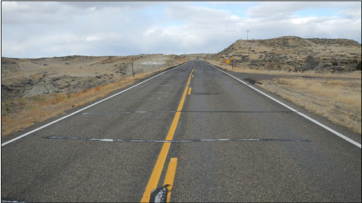
PHOTO 10: RP 4.7 LOOKING NORTH – RECENT SLIDE AREA
