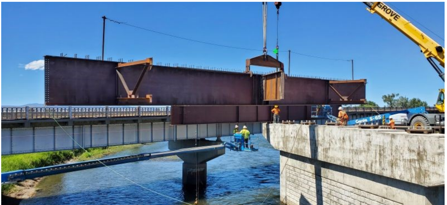
Construction crews set beams for a new bridge crossing the Missouri River as part of the Toston Structures Project (US Highway 287) in 2020.
