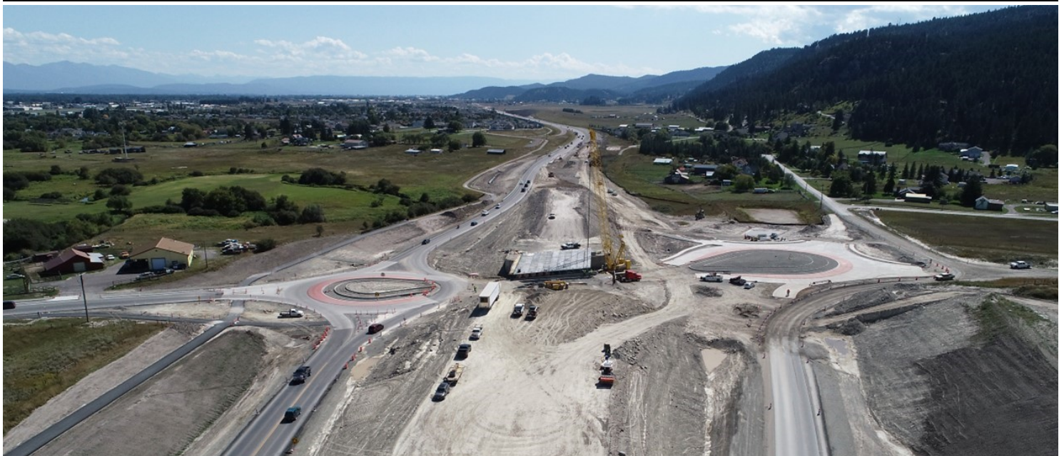
Drone footage of Foy's Lake Road construction—part of the Kalispell Bypass—in 2021 in Kalispell, Mont.
