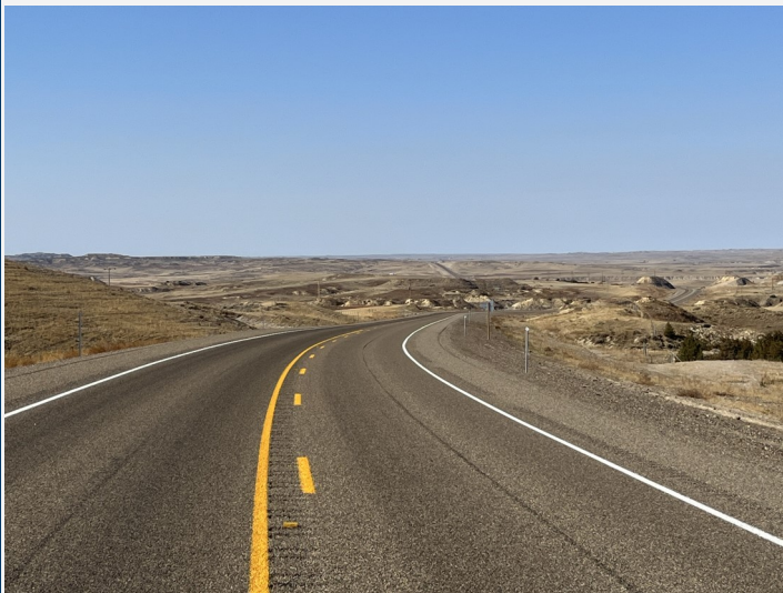
The project was completed in 2022, with improvements to MT 200 that include rumble strips, widened shoulders and pavement markings (as shown in the picture above).
